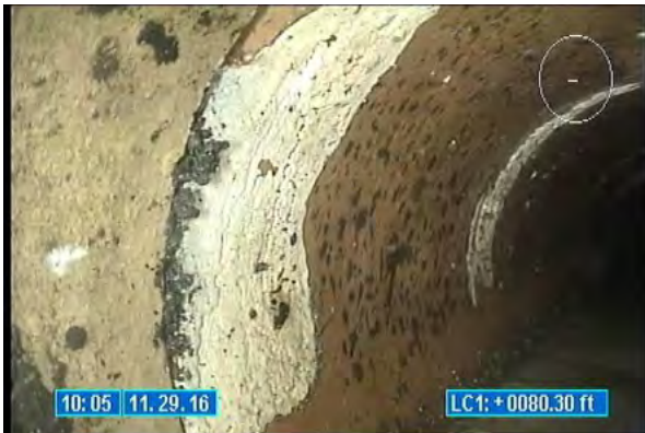
3940_129a0731-f7e2-4910-ba05-2e5cc384c581.jpg, 00:00:14, 80.30 Deposits Attached Encrustation, from 08 to 04 o'clock, within 8 inch
