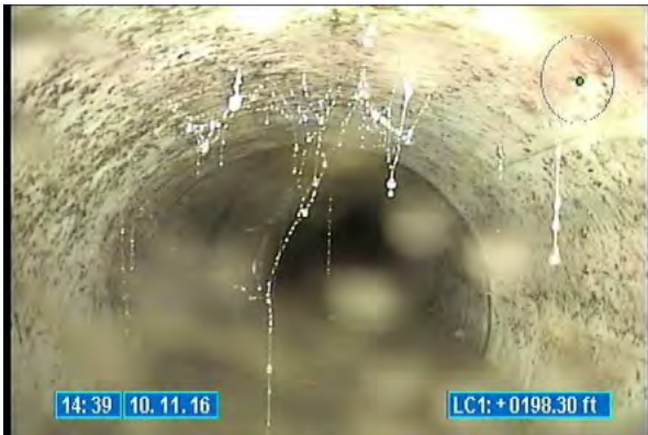
3540_bcc1d1e8-51fb-451f-98b3-fa8b5742b03a.jpg, 00:00:32, 198.30 Water Level, Sag in pipe
