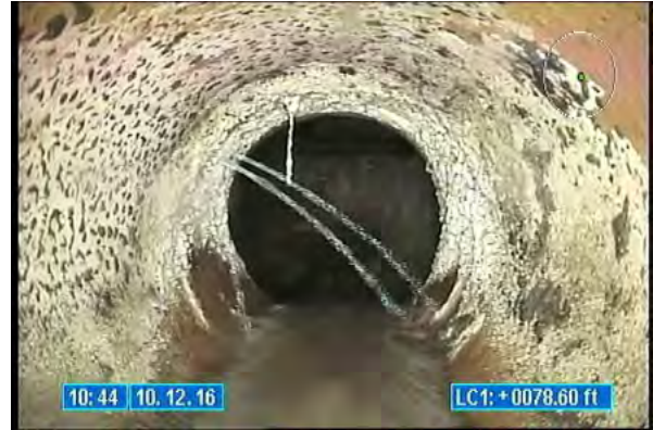
3650_faf91cee-bd8c-4089-ad56-365ded1ebc57.jpg, 00:00:09, 78.60 Deposits Attached Encrustation, from 08 to 04 o'clock
