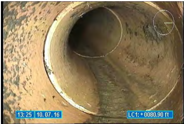
3410_6196f058-e4d7-438a-8090-18ca0d2f755e.jpg, 00:00:14, 80.90 Tap Factory Made, at 03 o'clock, 6 inch dim
