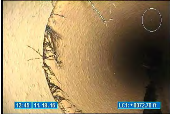
3210_84c6fb8e-967e-4f00-a594-74989724a46b.jpg, 00:00:06, 72.70 Roots Fine Joint, from 08 to 03 o'clock, within 8 inch
