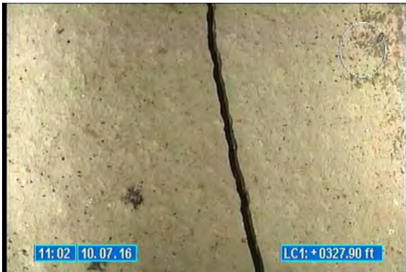
3500_aa56e070-7e1b-4338-9f31-8f10eacbe31d.jpg, 00:00:42, 327.90 Fracture Circumferential, from 12 to 12 o'clock, within 8 inch
