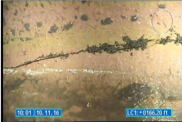
3120_473d7112-31cc-4f3e-9252-d5c1a0e9851c.jpg, 00:00:28, 166.20 Crack Longitudinal, at 05 o'clock, within 8 inch
