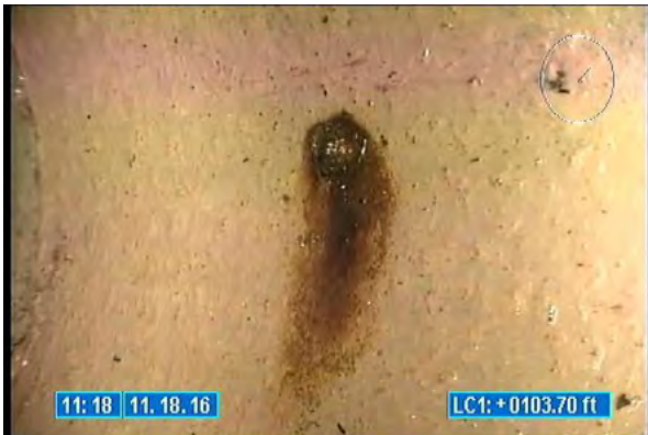
3430_ca148b6c-2142-48b7-b9f2-8bb025d9bb62.jpg, 00:00:09, 103.70 Infiltration Stain, at 02 o'clock, within 8 inch
