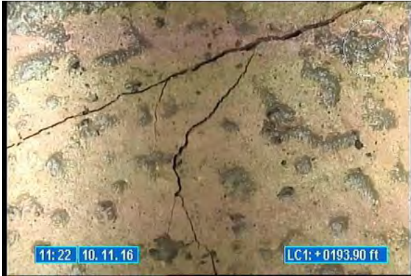
3150_6bbd1b71-ce94-4394-b229-f422db4be8c7.jpg, 00:00:20, 193.90 Fracture Multiple, from 10 to 02 o'clock
