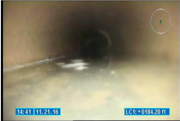
3750_f2406eab-b7cb-439b-bf45-2cf79c0e5348.jpg, 00:00:20, 184.20 Water Level, Sag in pipe
