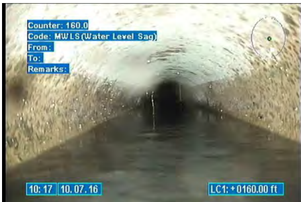
3520_6421cf81-c6b6-4142-9957-84e826cdd9fa.jpg, 00:00:31, 160.00 Water Level, Sag in pipe
