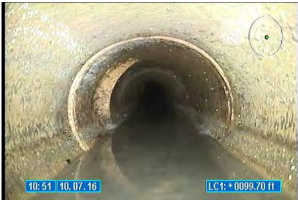
3500_9bddd870-38f8-4e75-954f-bfc94736aded.jpg, 00:00:14, 99.70 Deposits Settled Gravel, at 06 o'clock
