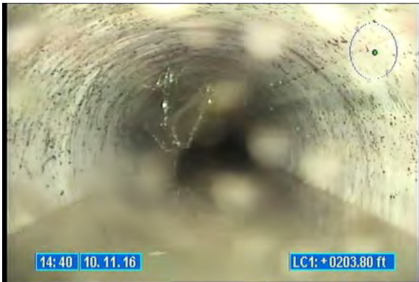
3540_7e5730d1-17f3-4f77-8209-9085fc4e16b1.jpg, 00:00:34, 203.80 Water Level, Sag in pipe, S01
