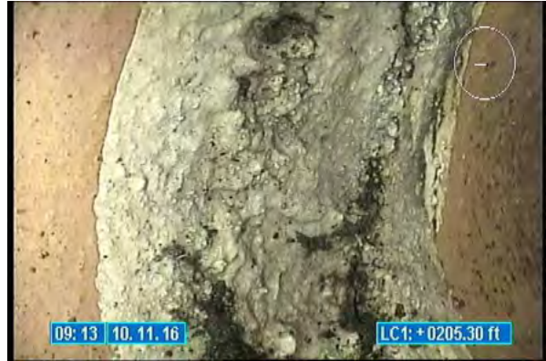
3100_1f3d131f-cb32-4f3e-aae5-099d3a2d31aa.jpg, 00:00:25, 205.30 Deposits Attached Encrustation, from 08 to 04 o'clock, within 8 inch
