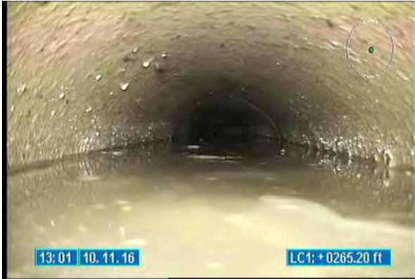
3620_5ca9c15b-4ba0-49a7-a704-966908a6174c.jpg, 00:00:43, 265.20 Water Level, Sag in pipe
