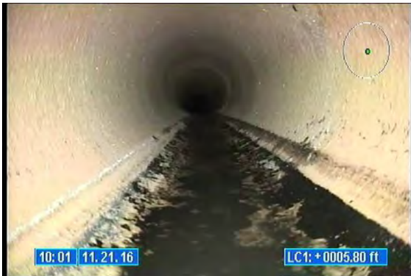
3450_fdf8f00a-04ff-43f0-a372-9ae19c53431a.jpg, 00:00:02, 5.80 Water Level, Sag in pipe
