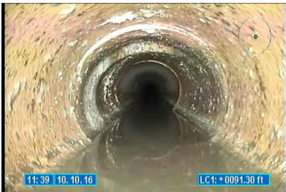
3300_1eda52d7-b403-4e94-afb8-8ad340ca6450.jpg, 00:00:18, 91.30 Water Level, Sag in pipe
