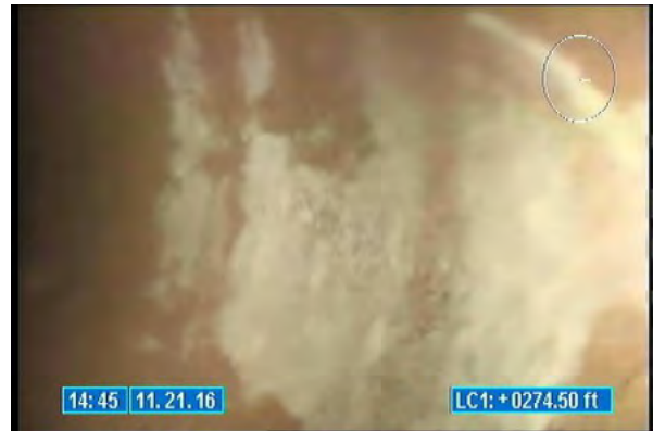
3750_ddb3d5bf-6582-4273-9633-dc0e8626dae2.jpg, 00:00:30, 274.50 Deposits Attached Encrustation, from 12 to 05 o'clock
