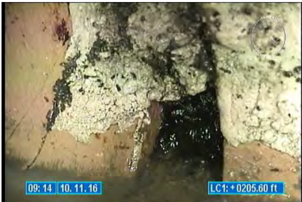
3100_be809c78-c976-488b-93fe-8730951ef095.jpg, 00:00:26, 205.60 Infiltration Stain, from 08 to 04 o'clock, within 8 inch
