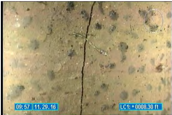
3940_68c20f11-1fbc-4ffe-903a-c830a3454888.jpg, 00:00:01, 8.30 Fracture Circumferential, from 07 to 05 o'clock
