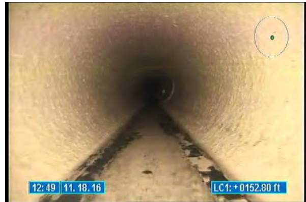
3210_b82d1017-3f6c-492a-ba4e-911ede1d330b.jpg, 00:00:15, 152.80 Water Level, Sag in pipe
