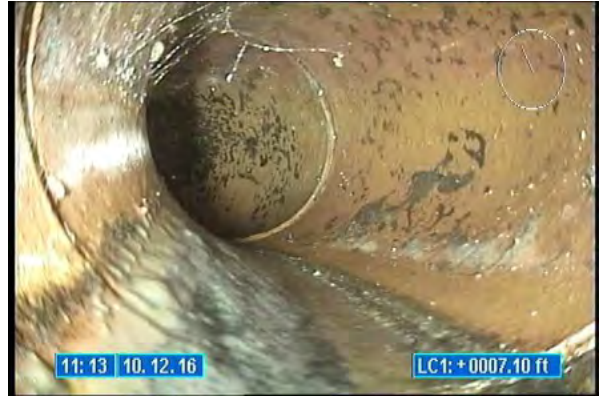
3690_4fdeeb1d-c919-4359-a93b-6589e505dbbd.jpg, 00:00:07, 7.10 Tap Factory Made Active, at 11 o'clock, 6 inch dim
