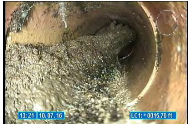
3410_a4f77346-3e91-47cc-9528-2d81957bf81e.jpg, 00:00:05, 15.70 Tap Factory Made, at 02 o'clock, 6 inch dim
