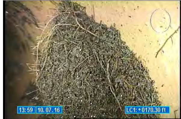
3230_fd13d62c-1727-42d8-b895-287d885ee66a.jpg, 00:00:18, 170.30 Roots Medium Joint, from 02 to 04 o'clock, within 8 inch
