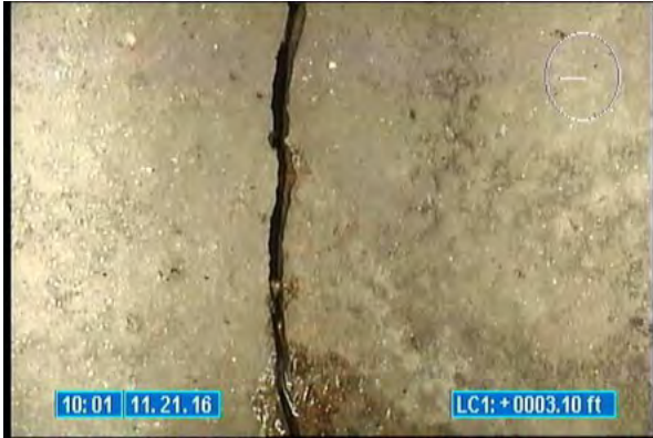
3450_3264803d-c945-45ae-9973-4e7ff883be20.jpg, 00:00:01, 3.10 Fracture Circumferential, from 12 to 12 o'clock
