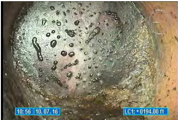
3500_1f927df7-ee92-477d-af5b-6cbdaeb67f57.jpg, 00:00:28, 194.00 Tap Factory Made Capped, at 09 o'clock, 6 inch dim
