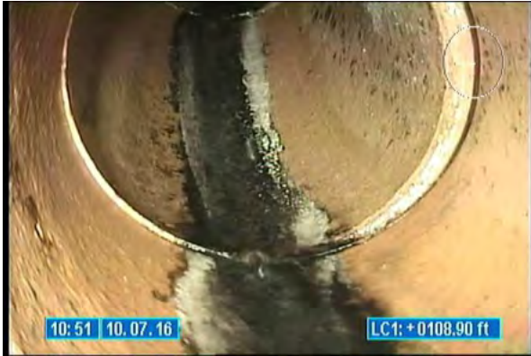
3500_0feed9e5-7dcf-4270-ad80-489e804d088a.jpg, 00:00:16, 108.90 Tap Factory Made Active, at 10 o'clock, 6 inch dim
