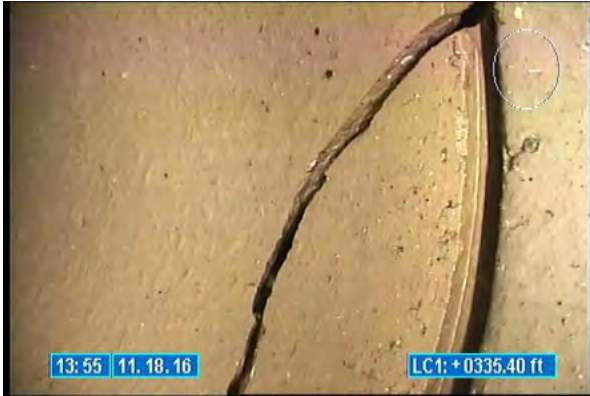
3180_3d623281-4522-4d8d-9a88-6ebf4609093e.jpg, 00:00:30, 335.40 Fracture Circumferential, from 02 to 05 o'clock, within 8 inch
