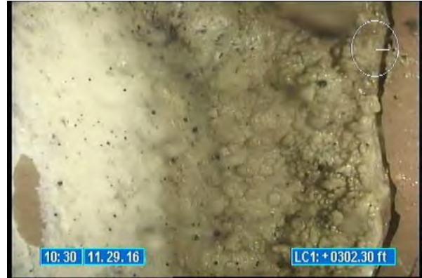
3940_cbbded02-768b-4075-b8e2-c97fd2ca415e.jpg, 00:01:01, 302.30 Deposits Attached Encrustation, from 12 to 05 o'clock
