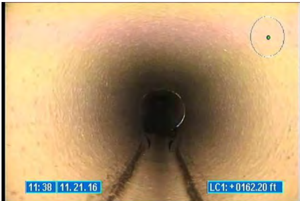
3290_5cc72e0b-bdb3-44ef-ac7e-33291cbb2398.jpg, 00:00:22, 162.20 Water Level, Sag in pipe, F01
