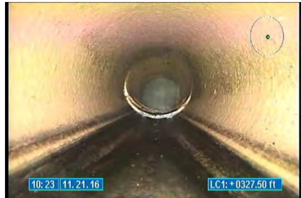
3450_ad1b9ddb-6e4a-49a0-9b10-f1b8d3792dd6.jpg, 00:00:41, 327.60 Water Level, Sag in pipe
