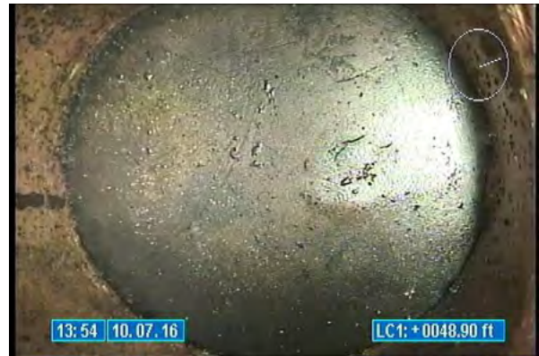
3230_397ab0d6-4729-425a-aeb4-0b4ac2f9a15e.jpg, 00:00:06, 48.90 Tap Factory Made Capped, at 03 o'clock, 6 inch dim
