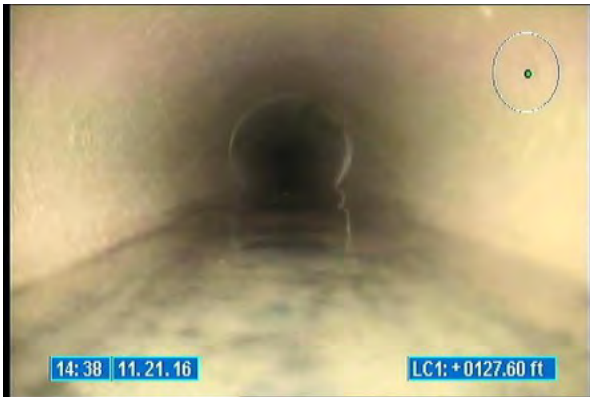
3750_0c70e91d-c3a3-416b-a575-b42d2c49a80a.jpg, 00:00:16, 127.60 Water Level, Sag in pipe
