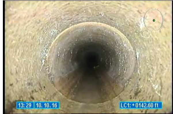
3310_afeb7514-12db-426e-b58b-aeef781a7856.jpg, 00:00:23, 142.90 Water Level, Sag in pipe, F01
