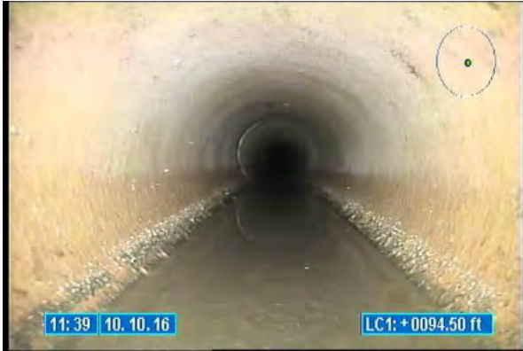
3300_1aa6e0d0-67d4-4c46-9ec8-b314eb79eab7.jpg, 00:00:20, 94.40 Water Level, Sag in pipe
