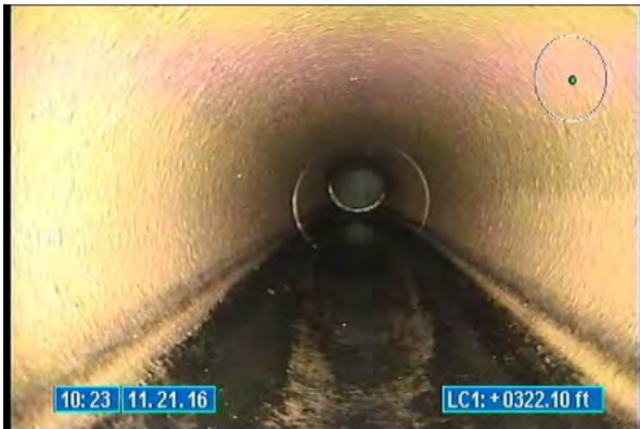
3450_b4276123-3d9e-4138-a4f5-0c552775d772.jpg, 00:00:40, 322.20 Water Level, Sag in pipe
