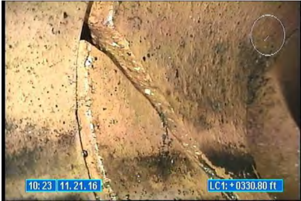
3450_579d77ce-fcda-4728-82f5-56cc72045e34.jpg, 00:00:42, 330.80 Broken, from 04 to 08 o'clock, within 8 inch
