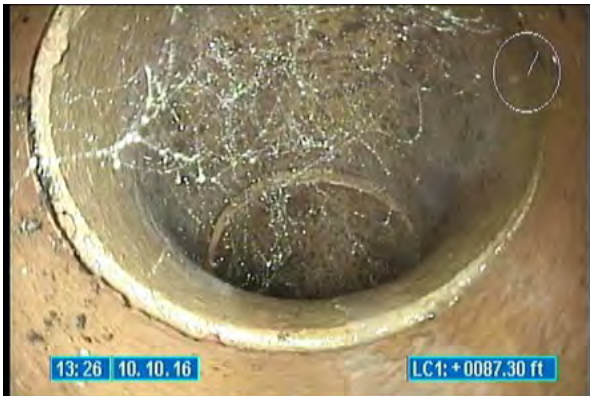
3310_2f9f28bc-cc03-4786-a923-19f78c3ec0d8.jpg, 00:00:17, 87.30 Tap Factory Made, at 02 o'clock, 6 inch dim
