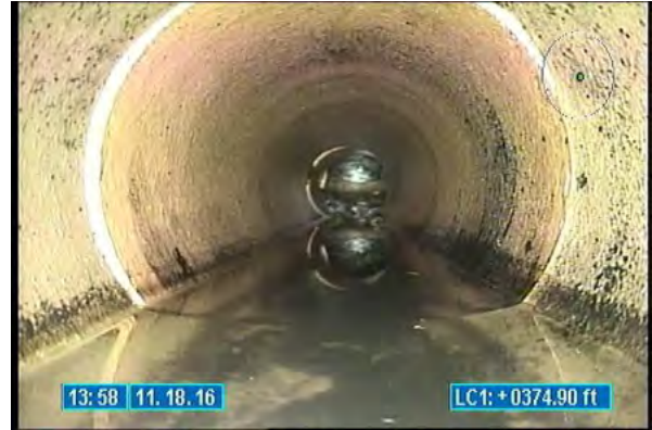
3180_938b4587-599c-4803-b4c6-61f267103f0f.jpg, 00:00:35, 374.90 Water Level, Sag in pipe
