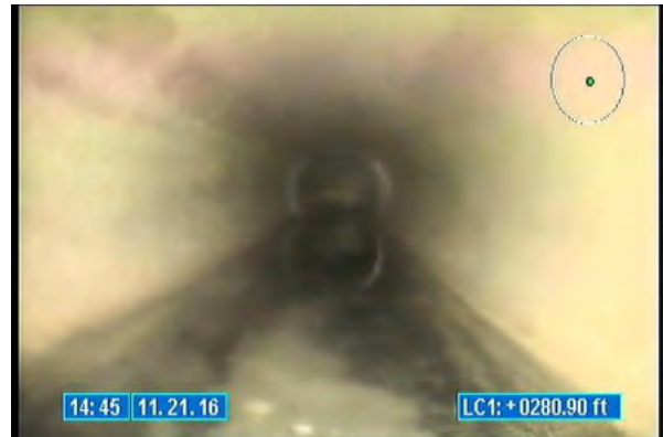
3750_e197e2af-7df5-4ce7-b655-b41d2b3c54b9.jpg, 00:00:31, 280.90 Water Level, Sag in pipe
