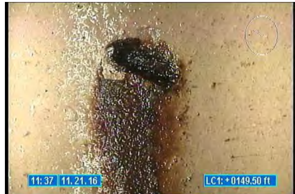
3290_b5f6115a-72e6-42fe-9158-9eccaed32fef.jpg, 00:00:20, 149.50 Infiltration Stain, at 10 o'clock
