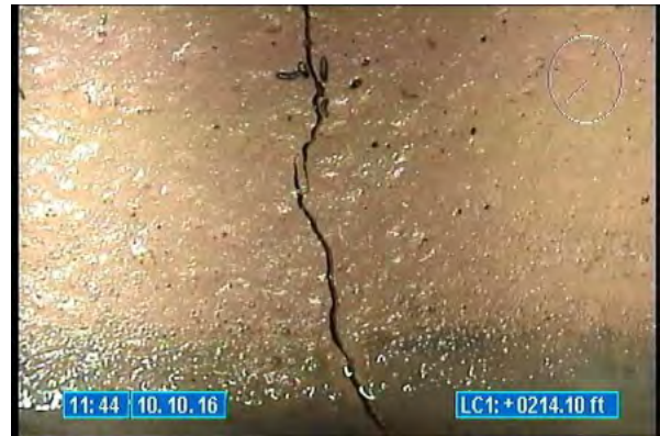
3300_fcb360f1-c01b-47cc-91e4-4ddb1f4e774c.jpg, 00:00:31, 214.10 Fracture Circumferential, from 12 to 12 o'clock
