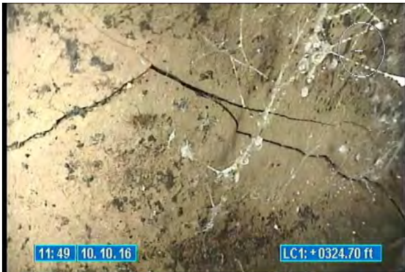
3300_1d73a4d3-75e5-47c9-9ca7-c5686586b554.jpg, 00:00:44, 324.70 Fracture Multiple, from 12 to 12 o'clock, within 8 inch
