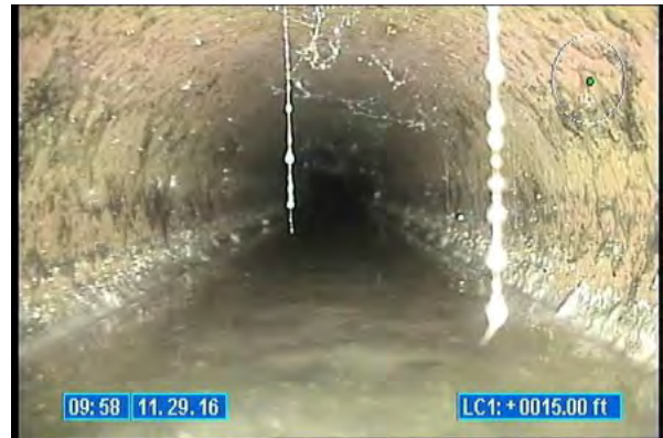
3940_7a555b58-d1c2-438b-9be4-90eac712b26f.jpg, 00:00:03, 15.00 Water Level, Sag in pipe
