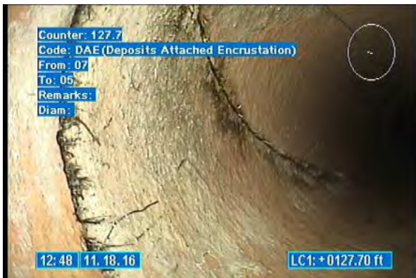
3210_a21ae127-3283-46f9-908a-a4838daf3ae5.jpg, 00:00:12, 127.70 Roots Fine Joint, from 07 to 05 o'clock, within 8 inch
