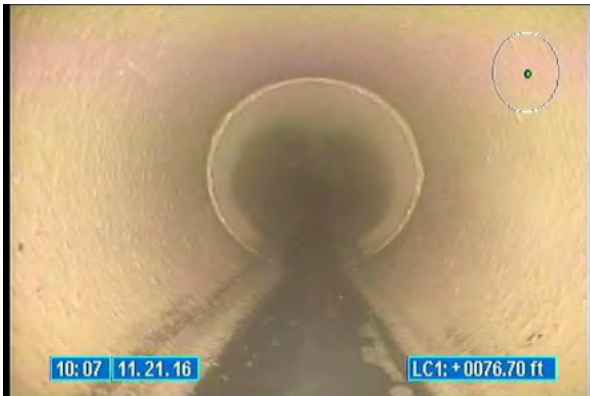
3450_58bad82b-8685-404b-b498-f9829c9e0903.jpg, 00:00:10, 76.60 Water Level, Sag in pipe
