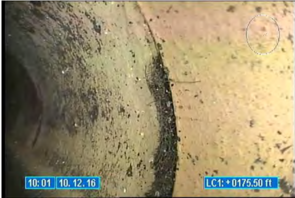
3560_536bb00d-7f45-424a-aa6c-1ce4ee9b7793.jpg, 00:01:21, 175.50 Roots Fine Joint, from 08 to 04 o'clock, within 8 inch
