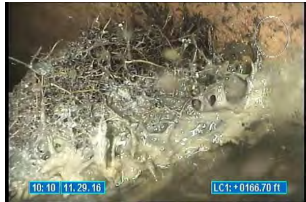
3940_a4acd987-6ac7-439c-b7d0-7c2e0a40698a.jpg, 00:00:27, 166.70 Roots Medium Joint, at 05 o'clock, within 8 inch
