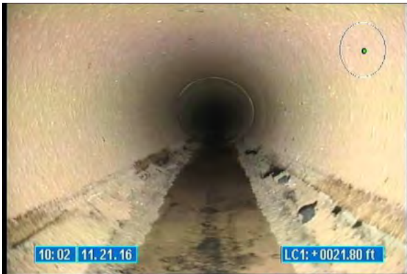
3450_5d941d3e-c575-4547-8193-08da863161d1.jpg, 00:00:04, 21.80 Water Level, Sag in pipe
