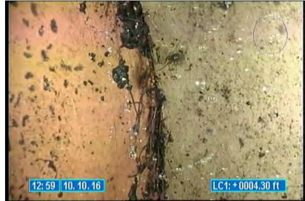
3310_01a686ed-3bd7-4dd4-9578-9af21579e50d.jpg, 00:00:01, 4.30 Roots Fine Joint, from 08 to 04 o'clock, within 8 inch
