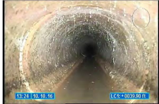
3310_f2f4d776-9274-4cf6-b513-adcc4e35c9d1.jpg, 00:00:13, 40.20 Water Level, Sag in pipe
