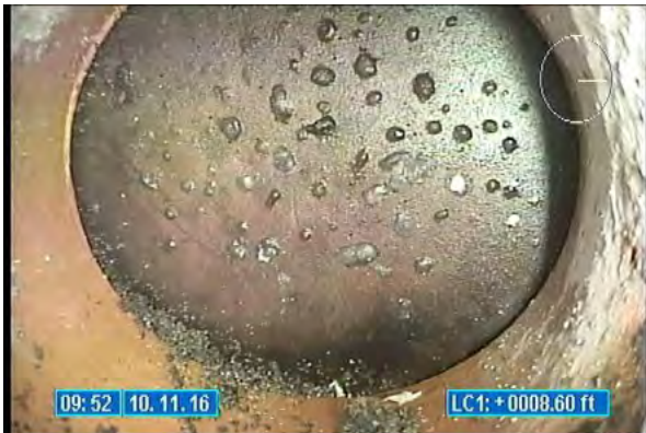
3120_4fd40679-8bb7-41c0-880f-5f40e0fc5836.jpg, 00:00:06, 8.60 Tap Factory Made Capped, at 03 o'clock, 6 inch dim
