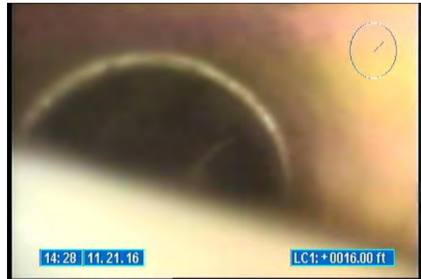
3750_071ceb18-8a48-45ce-9011-77878d866850.jpg, 00:00:03, 16.00 Tap Factory Made, at 03 o'clock, 6 inch dim
