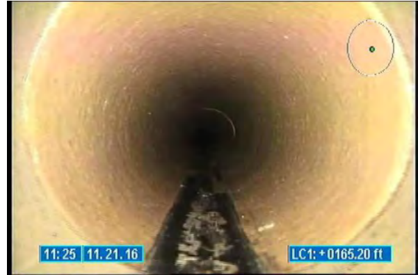
3280_009b5d4a-e3d6-43b2-89cd-0a2558919bb2.jpg, 00:00:15, 165.50 Water Level, Sag in pipe, F01
