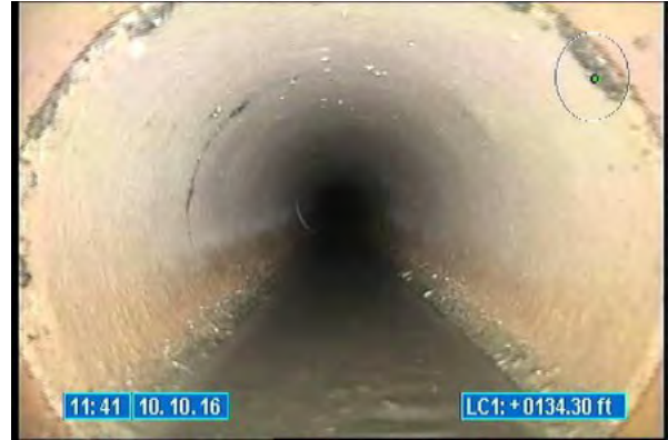
3300_aa5a4151-93df-4096-9627-5a1e6c386363.jpg, 00:00:24, 133.70 Water Level, Sag in pipe
