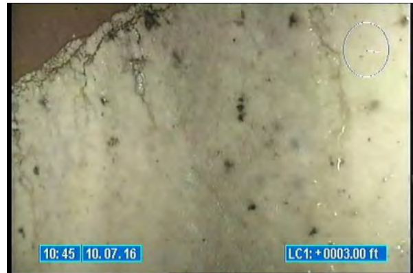
3500_f5c833a9-0544-4b7e-b067-4d8335f0c706.jpg, 00:00:02, 3.00 Deposits Attached Encrustation, from 02 to 05 o'clock, within 8 inch
