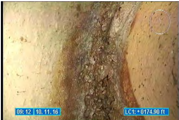
3100_126885b8-b118-4739-8b7d-63b0c551ba99.jpg, 00:00:21, 174.90 Deposits Attached Encrustation, from 08 to 04 o'clock, within 8 inch
