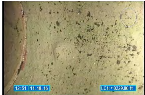
3210_0b94685d-56aa-4103-8179-6b9365832b81.jpg, 00:00:20, 229.00 Buckling Dimpling, at 02 o'clock
