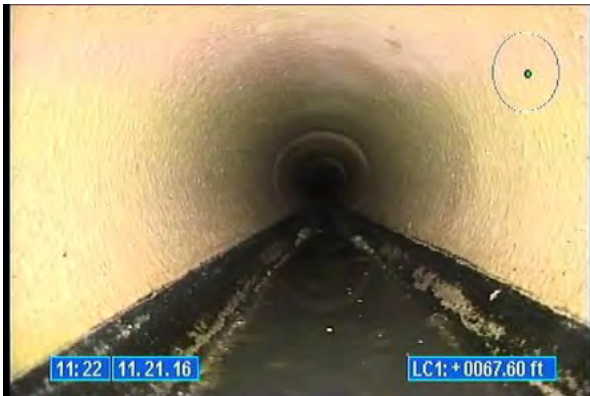
3280_b011b40c-24d9-4069-bf29-2493745224ea.jpg, 00:00:09, 67.60 Water Level, Sag in pipe
