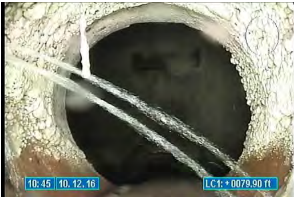
3650_44c3b86d-0e71-469f-a174-3ccdc4d8be02.jpg, 00:00:12, 79.90 Infiltration Gusher, from 09 to 03 o'clock
