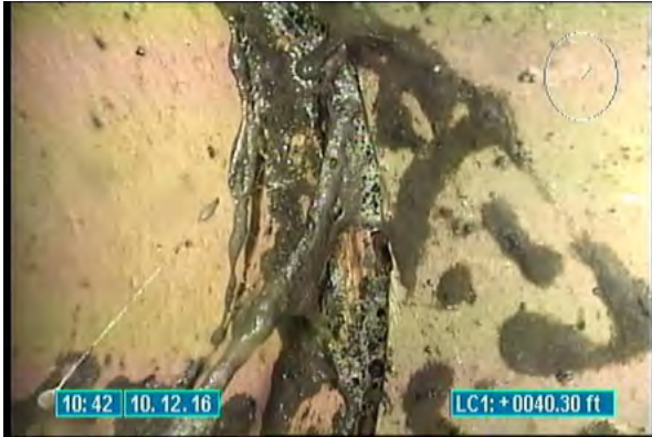
3650_58e1a8c9-11aa-4433-96f4-61edb275afed.jpg, 00:00:05, 40.30 Roots Fine Joint, at 02 o'clock, within 8 inch
