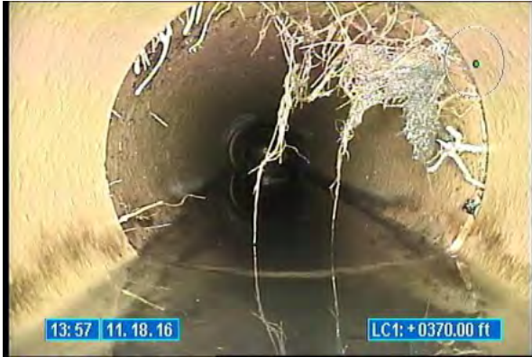
3180_4770dd6f-5d3e-4818-84ca-6e64f3b5b13d.jpg, 00:00:34, 370.00 Roots Medium Joint, from 08 to 04 o'clock, within 8 inch
