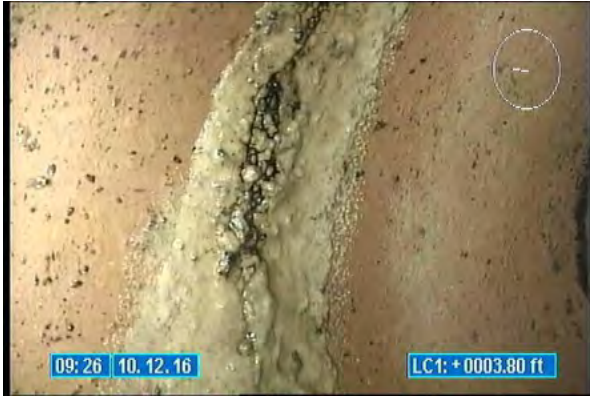
3560_2af37fd7-f3a4-4382-b81c-5e3e9b3d3362.jpg, 00:00:02, 3.80 Deposits Attached Encrustation, from 08 to 04 o'clock, within 8 inch
