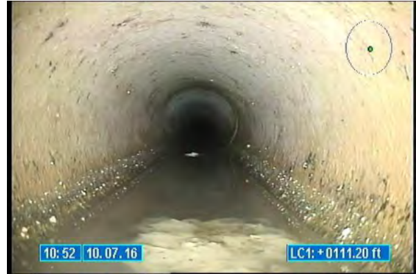
3500_5e8cec27-0618-4e14-9229-ab5fb6dd3725.jpg, 00:00:17, 111.20 Deposits Settled Gravel, at 06 o'clock
