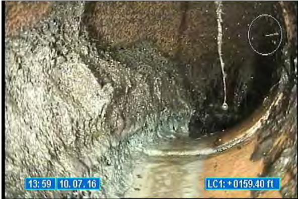
3230_0545705b-c7f8-4a6c-9083-c6562070dff1.jpg, 00:00:17, 159.40 Tap Factory Made, at 03 o'clock, 6 inch dim
