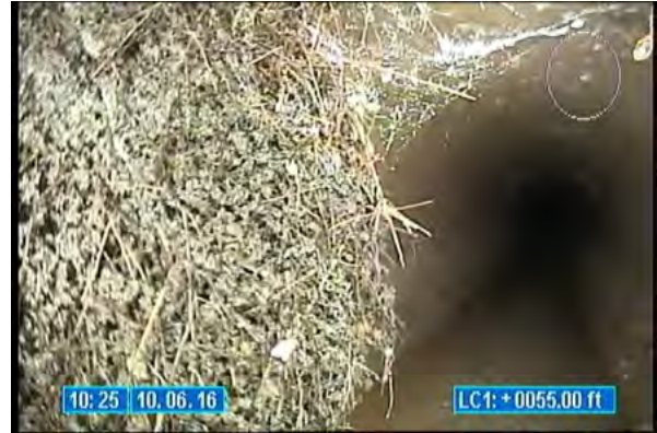
3010_751128d3-42f6-48c3-9afd-b3003edf7118.jpg, 00:00:06, 55.00 Roots Medium Joint, from 08 to 04 o'clock, within 8 inch
