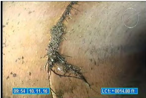
3120_22a49c61-1520-4352-afe6-b94d8852a813.jpg, 00:00:11, 14.80 Roots Fine Joint, at 08 o'clock, within 8 inch
