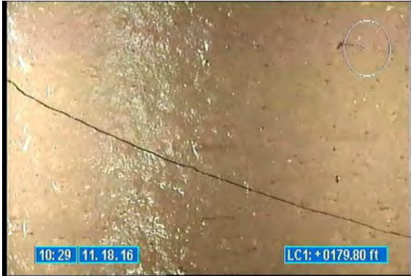
3350_10ed5cdf-cfb9-4fb3-a910-09fced922627.jpg, 00:00:19, 179.80 Crack Longitudinal, at 10 o'clock, within 8 inch
