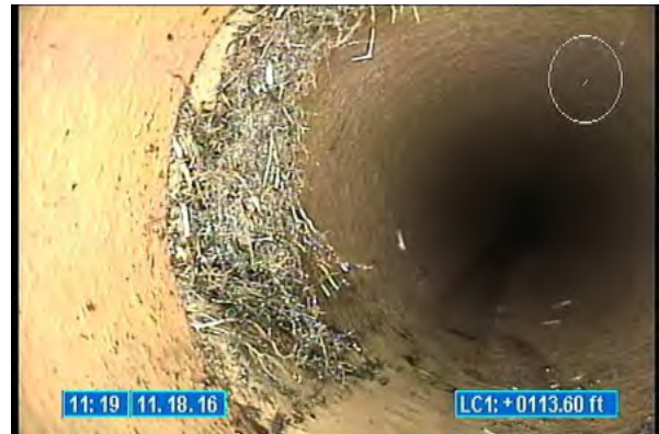
3430_2e251305-ded0-4791-ba00-a20cb20fea52.jpg, 00:00:11, 113.60 Roots Medium Joint, from 07 to 05 o'clock, within 8 inch
