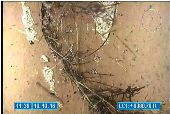
3300_1b15b9a4-91bd-4969-ac58-51636d15e050.jpg, 00:00:16, 80.70 Fracture Circumferential, from 08 to 04 o'clock, within 8 inch
