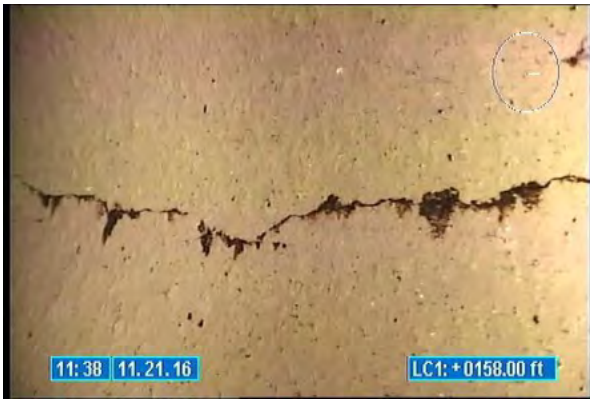
3290_cf4b19d1-138e-4822-a6dc-40a03134df0f.jpg, 00:00:21, 158.00 Crack Longitudinal, at 03 o'clock
