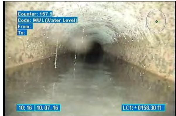
3520_3ff49abc-81a1-46de-bfb1-f982a0dd4067.jpg, 00:00:30, 157.50 Water Level
