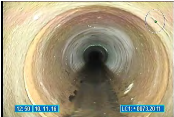
3620_e1875589-e238-4d30-b85c-cfeadf070732.jpg, 00:00:15, 73.20 Infiltration Runner, at 12 o'clock, within 8 inch
