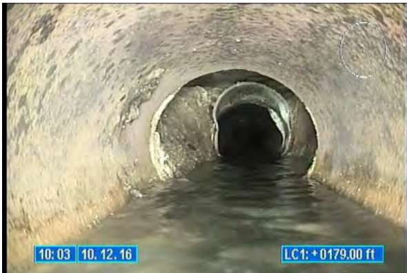
3560_88eb8ff0-6b15-4504-b1f2-8c59c1e0b5e9.jpg, 00:01:26, 179.00 Deposits Settled Gravel, at 06 o'clock
