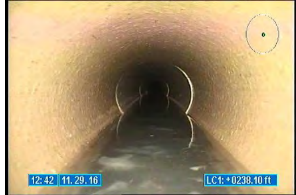
3660_7bd1882f-311f-445e-bc92-95f43a5c2824.jpg, 00:00:15, 238.40 Water Level, Sag in pipe, S01
