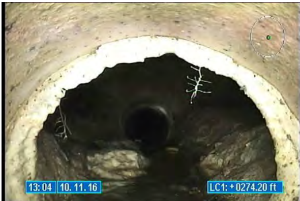
3620_a5b88384-b860-4a3a-aba3-ecabf1a748d0.jpg, 00:00:50, 274.20 Deposits Attached Encrustation, from 08 to 04 o'clock, within 8 inch
