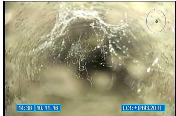
3540_51f9942c-f162-4767-b372-0236e3972883.jpg, 00:00:30, 193.20 Water Level, Sag in pipe
