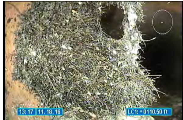
3190_7ce82c0d-ef6b-4242-af58-d43d1ef84ffa.jpg, 00:00:13, 110.50 Roots Medium Joint, from 07 to 05 o'clock, within 8 inch
