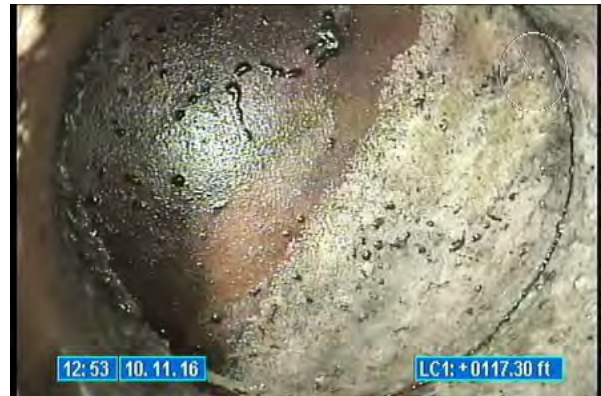
3620_68e30b90-bcb9-4ab3-9478-b97c111b0d0c.jpg, 00:00:23, 117.30 Tap Factory Made Capped, at 10 o'clock, 6 inch dim
