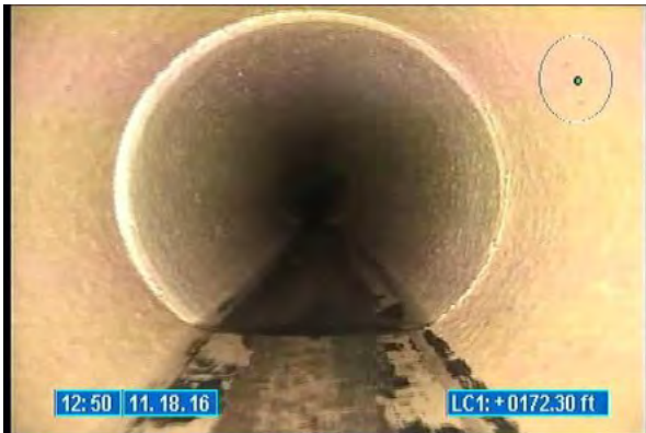
3210_122e696a-02c5-431b-80bd-561da0c55d33.jpg, 00:00:16, 172.70 Water Level, Sag in pipe
