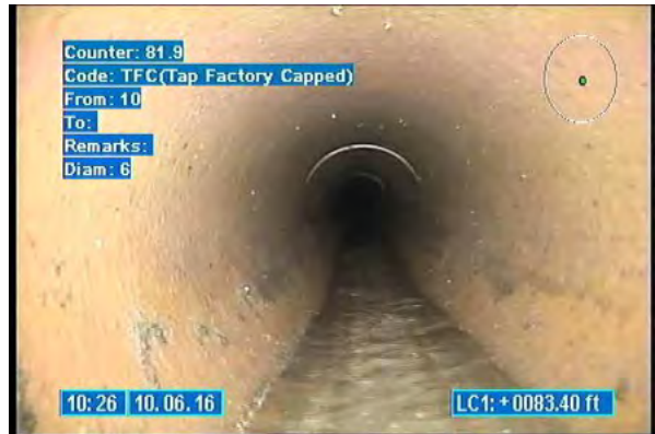
3010_ca52b791-b218-4710-b76c-161c7b6f11d1.jpg, 00:00:10, 83.30 Water Level, Sag in pipe
