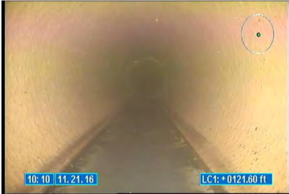
3450_5fbcd45a-f211-4a3d-81de-89cf53e2b99c.jpg, 00:00:16, 121.60 Water Level, Sag in pipe
