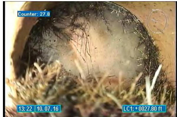
3410_de58cd3c-b749-4b93-9e9e-7daf0a1ef35b.jpg, 00:00:08, 27.80 Tap Factory Made Capped, at 10 o'clock, 6 inch dim
