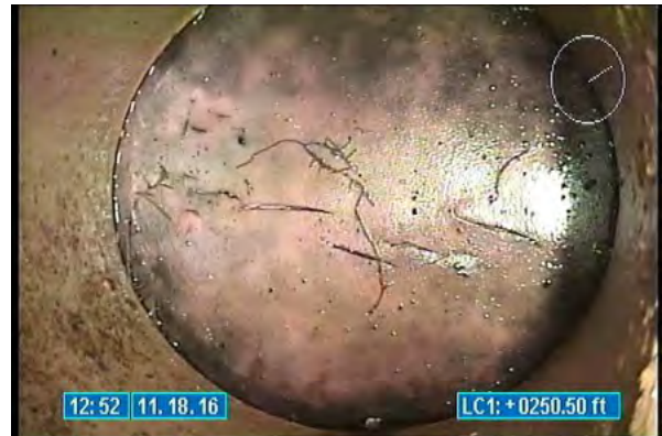
3210_09f424ae-94f7-41fe-b246-e3efc5865ccf.jpg, 00:00:22, 250.50 Tap Factory Made Capped, at 02 o'clock, 6 inch dim
