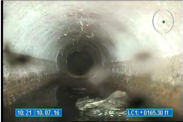
3520_e76b623f-05be-4179-b3e2-d42d17bc39c4.jpg, 00:00:42, 165.30 Deposits Settled Fine, at 06 o'clock, within 8 inch
