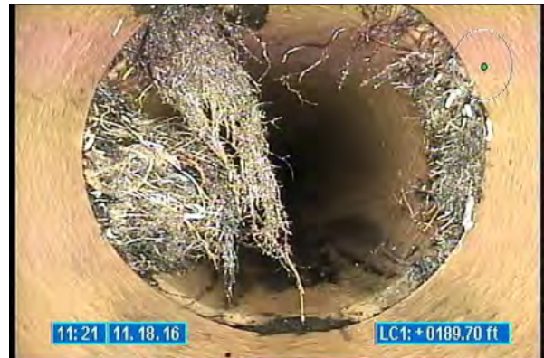
3430_47eec5e2-b142-46a1-8ef3-439f8dcc7568.jpg, 00:00:17, 189.70 Roots Medium Joint, from 07 to 05 o'clock, within 8 inch
