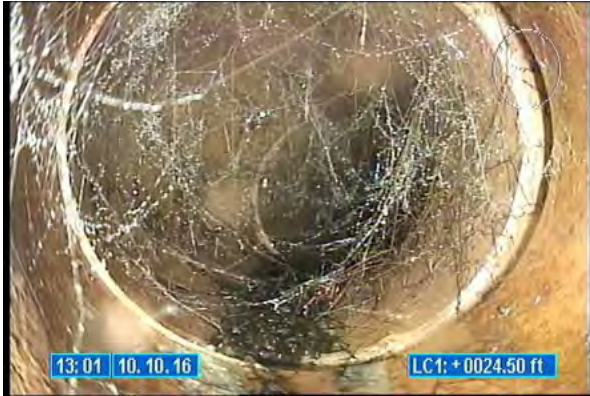
3310_6f7dcc97-8329-4dd8-92f7-4a9444625a5f.jpg, 00:00:05, 24.50 Tap Factory Made, at 09 o'clock, 6 inch dim
