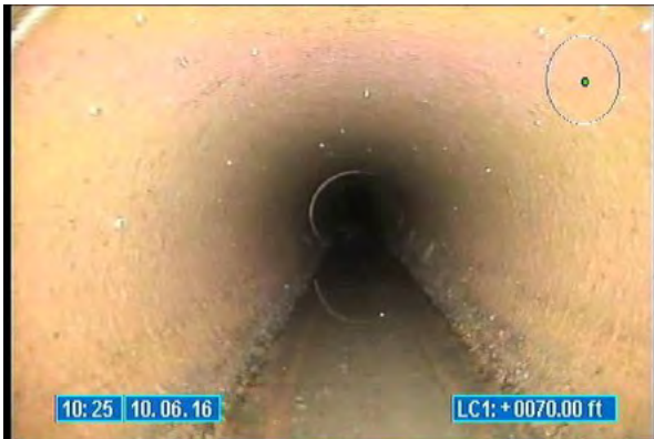
3010_63e467a3-424c-4770-a06d-634772caeca7.jpg, 00:00:08, 70.10 Water Level, Sag in pipe
