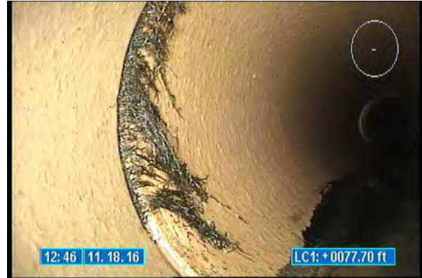
3210_9fd843ab-a749-499a-995a-de4c2aa5909a.jpg, 00:00:07, 77.70 Roots Fine Joint, from 08 to 04 o'clock, within 8 inch
