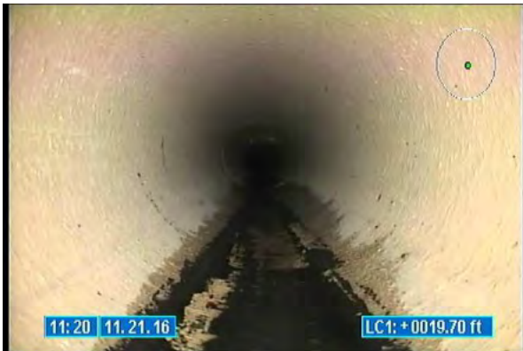
3280_5dc0ad9e-3fc3-439a-9e3a-9a0a63ad9319.jpg, 00:00:03, 19.70 Water Level, Sag in pipe
