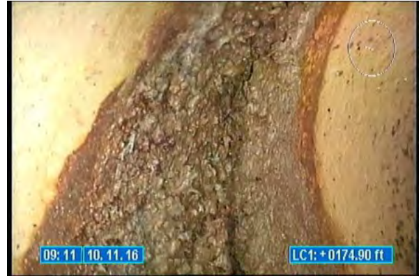
3100_a5f4d119-d8fa-499c-9fef-dd2f408cc66b.jpg, 00:00:21, 174.90 Infiltration Stain, from 08 to 04 o'clock, within 8 inch
