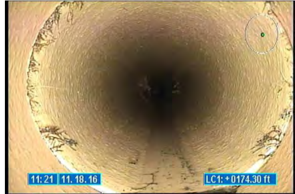
3430_5b2a1f56-7541-43cd-b776-b2754c747551.jpg, 00:00:16, 174.30 Roots Fine Joint, from 07 to 05 o'clock, within 8 inch
