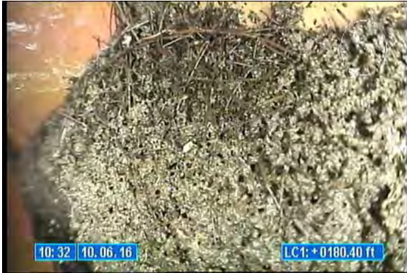
3010_42314b01-3a76-43fe-84ee-9549a578888e.jpg, 00:00:23, 180.40 Roots Medium Joint, at 04 o'clock, within 8 inch
