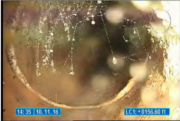
3540_d9e91841-c7e4-41be-b6ed-74417fc06717.jpg, 00:00:24, 156.60 Tap Factory Made, at 03 o'clock, 6 inch dim
