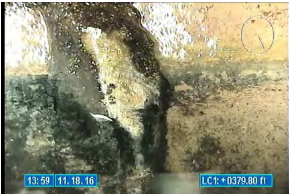
3180_65f45bc8-fb1f-4255-a36f-0d3407131711.jpg, 00:00:37, 379.80 Deposits Attached Encrustation, at 05 o'clock
