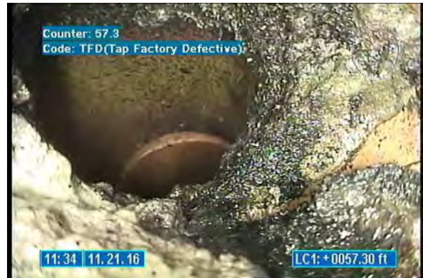
3290_16c9ffca-11fd-47bb-a9f4-cc59c1d6fd5c.jpg, 00:00:11, 57.30 Tap Factory Made Defective, at 10 o'clock, 6 inch dim
