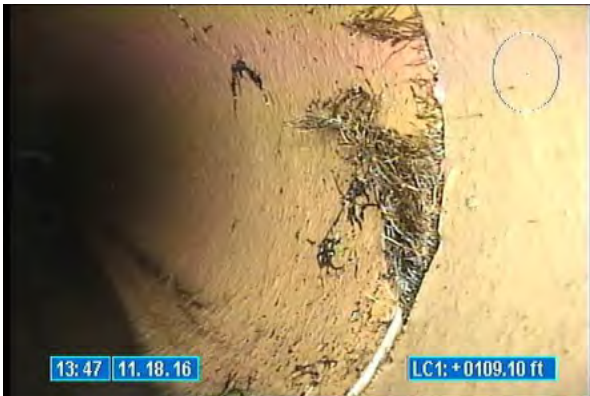
3180_b7c01b91-460f-4eaf-8bc6-01fbf76c6417.jpg, 00:00:09, 109.10 Roots Fine Joint, from 07 to 05 o'clock, within 8 inch
