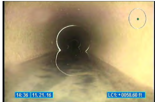
3750_1a126f4a-27c6-45ef-ae57-0bddb77d39f4.jpg, 00:00:09, 58.60 Water Level, Sag in pipe
