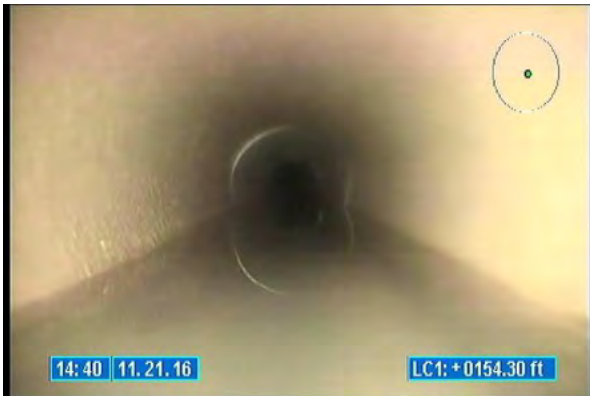
3750_f7642c40-d923-40d9-a2b8-0a90f2d3a65e.jpg, 00:00:19, 154.50 Water Level, Sag in pipe
