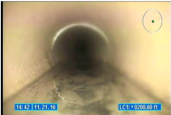
3750_9b6d8cf3-0fee-4f7c-946b-2f216e4f4000.jpg, 00:00:24, 208.60 Water Level, Sag in pipe
