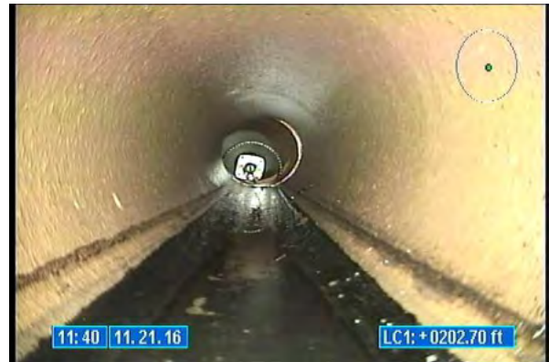
3290_bde35199-aa08-46ae-8707-fb2c4ccb3e51.jpg, 00:00:25, 202.70 Water Level, Sag in pipe
