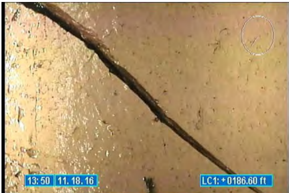
3180_a4654c5d-5d09-41be-9bb9-f11a07e34484.jpg, 00:00:17, 186.60 Fracture Circumferential, from 04 to 08 o'clock, within 8 inch
