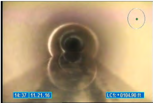
3750_3dbf86bf-d74c-411e-973a-05ee187260f2.jpg, 00:00:12, 104.90 Water Level, Sag in pipe
