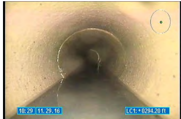
3940_1e2100f3-dcf3-4c6d-8142-0da4eba7e0aa.jpg, 00:00:59, 294.50 Water Level, Sag in pipe
