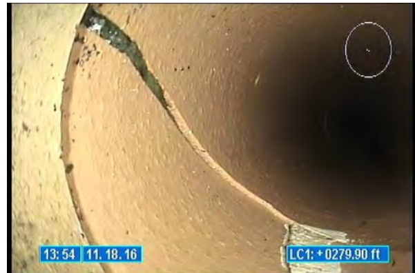
3180_42df683b-036e-4fc4-85a8-549118f48b47.jpg, 00:00:26, 279.90 Broken, from 05 to 12 o'clock, within 8 inch
