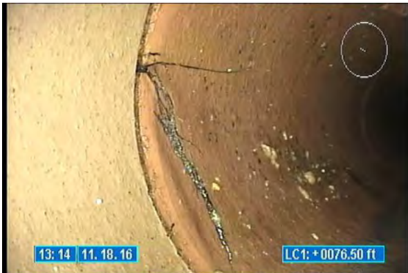
3190_7988817f-b799-4002-a455-2600bee9b824.jpg, 00:00:07, 76.50 Roots Fine Joint, at 10 o'clock, within 8 inch
