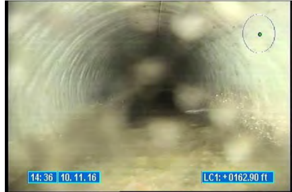
3540_93ffba7c-d0ab-404c-9d26-5e1a1a1c917b.jpg, 00:00:25, 162.70 Water Level, Sag in pipe
