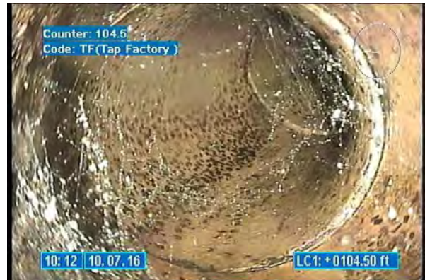
3520_e3018640-9b78-4726-9ca6-02e43c58551e.jpg, 00:00:20, 104.50 Tap Factory Made, at 09 o'clock, 6 inch dim
