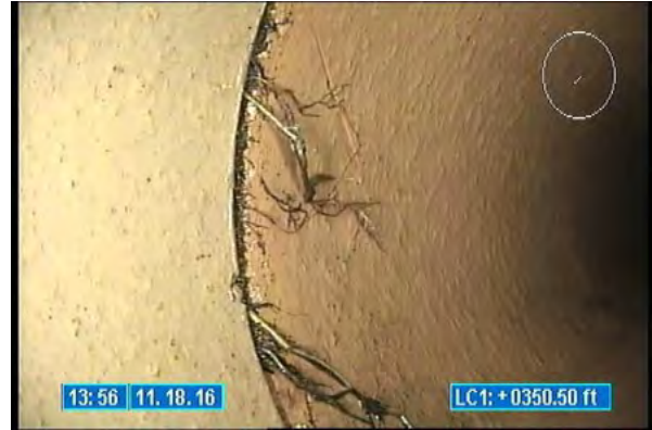
3180_58d2108e-8f40-4a4b-a730-e1e09d684d45.jpg, 00:00:31, 350.50 Roots Fine Joint, from 08 to 04 o'clock, within 8 inch
