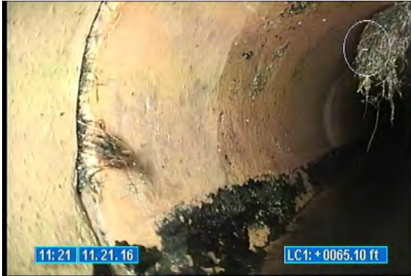
3280_8c517bf0-59b6-4aa0-aef6-d3ba022b38be.jpg, 00:00:07, 65.10 Roots Fine Joint, from 09 to 03 o'clock, within 8 inch
