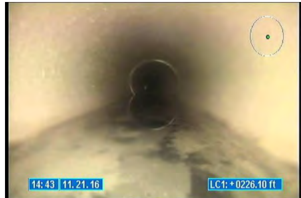
3750_81a0bd06-4620-472b-ba9e-b8a19559b8bf.jpg, 00:00:25, 226.10 Water Level, Sag in pipe
