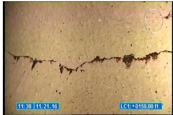
3290_9ab01cc8-2a8a-48d2-a25f-9d85badff1c9.jpg, 00:00:21, 158.00 Infiltration Stain, at 03 o'clock
