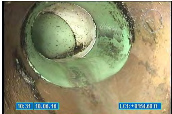
3010_28f04f93-77b3-4ebf-9b60-ee962aa2b304.jpg, 00:00:20, 154.60 Tap Factory Made Active, at 10 o'clock, 6 inch dim
