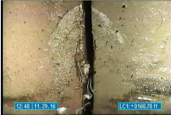
3660_421d952e-4a72-4d81-91a9-12ff4f27f839.jpg, 00:00:10, 160.70 Infiltration Runner, at 04 o'clock, within 8 inch
