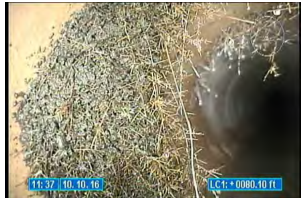
3300_b80f7030-6859-4075-9310-e8e08a257267.jpg, 00:00:14, 80.10 Roots Medium Joint, from 07 to 05 o'clock, within 8 inch
