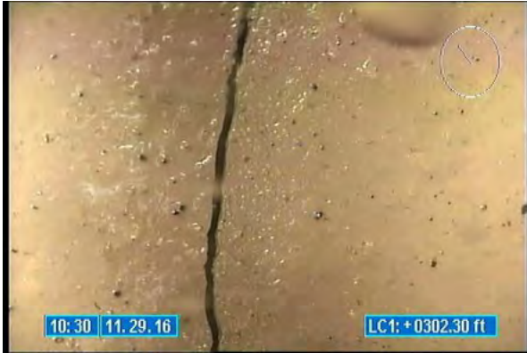
3940_679c5e36-e982-4847-a13d-f371584007f7.jpg, 00:01:00, 302.30 Fracture Circumferential, from 12 to 12 o'clock
