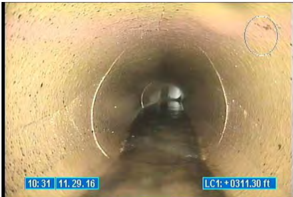
3940_eb26960e-462a-4ec1-80b0-02b41397219b.jpg, 00:01:03, 311.30 Fracture Longitudinal Hinge, 4, from 12 to 12 o'clock, within 8 inch
