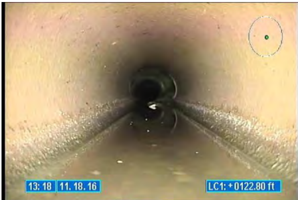
3190_e14e2bce-7740-456b-ae6d-46e16da74bbd.jpg, 00:00:16, 122.80 Water Level, Sag in pipe
