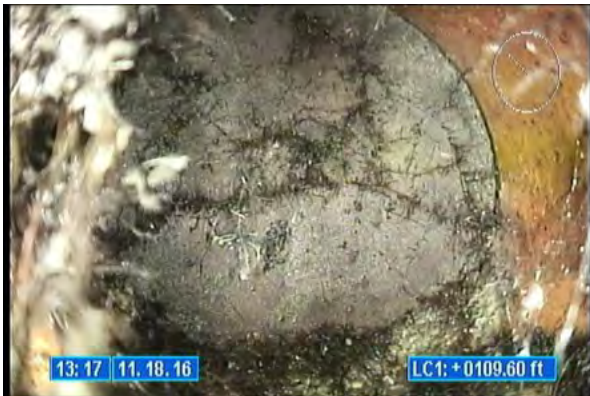
3190_c0490a67-de00-4b14-a125-6773a0bdebc0.jpg, 00:00:12, 109.60 Tap Factory Made Capped, at 10 o'clock, 6 inch dim
