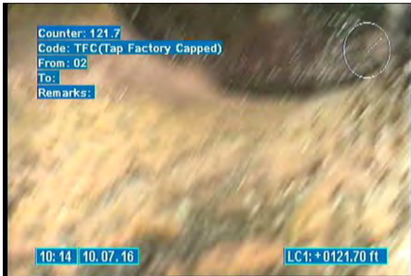
3520_540961d3-b2f6-4cd8-bd5d-c741a9d47ed4.jpg, 00:00:24, 121.70 Tap Factory Made Capped, at 02 o'clock, 6 inch dim
