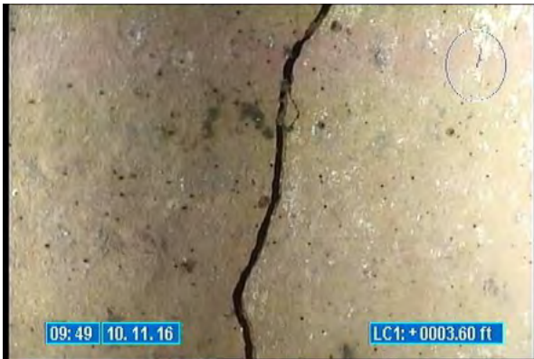
3120_b258ade0-c589-4721-a85f-1f38e4a9b977.jpg, 00:00:01, 3.60 Fracture Circumferential, from 12 to 12 o'clock
