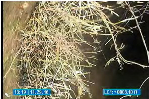
3870_1c268518-b998-4f22-b4d0-b8dd3a1ae3a0.jpg, 00:00:01, 3.10 Roots Medium Joint, from 08 to 04 o'clock, within 8 inch
