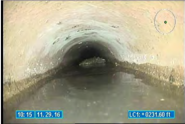
3940_e79fabd4-7a0b-454b-b0a0-564fb507b550.jpg, 00:00:38, 231.60 Obstacles Pipe Material, at 06 o'clock
