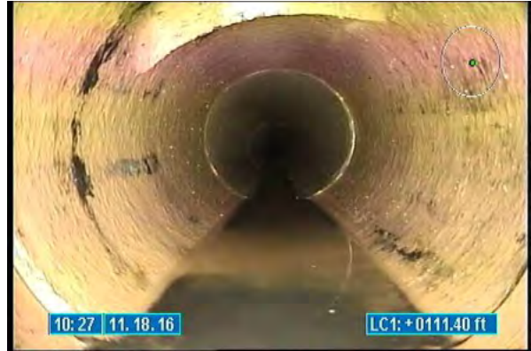
3350_2002798b-de82-48b5-abc4-df4d0890aa13.jpg, 00:00:13, 111.40 Water Level, Sag in pipe
