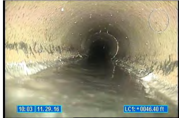
3940_3e67d28a-384e-4c20-87ef-d34d5f7bcb01.jpg, 00:00:09, 46.40 Deposits Settled Gravel, at 06 o'clock
