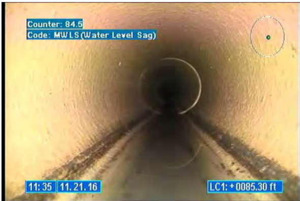
3290_0063699e-ca59-4180-ae2c-d333fe92194f.jpg, 00:00:13, 84.50 Water Level, Sag in pipe
