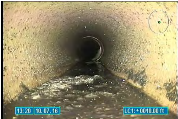
3410_792dcbe0-c089-4109-adaf-cbab90721ff6.jpg, 00:00:03, 10.00 Water Level, Sag in pipe
