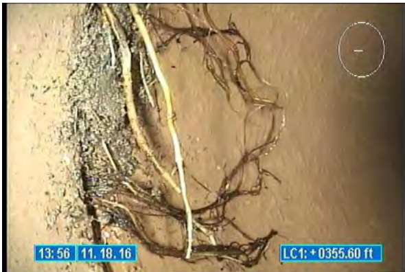
3180_180f1cb1-3673-4ae7-9915-e2ca436aec4e.jpg, 00:00:33, 355.60 Roots Fine Joint, from 09 to 03 o'clock, within 8 inch
