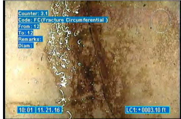
3450_6852d5a6-f71b-4114-b210-e91d0053aaf1.jpg, 00:00:01, 3.10 Infiltration Stain, from 06 to 09 o'clock
