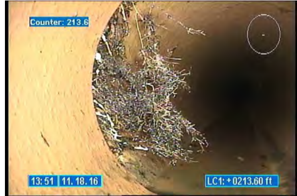
3180_0b801483-91c4-4278-bdaa-21aad5f9b092.jpg, 00:00:21, 213.60 Roots Medium Joint, from 07 to 05 o'clock, within 8 inch
