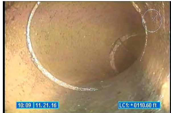
3450_67a4bcde-3bf4-46c5-9821-390852036a17.jpg, 00:00:14, 110.60 Tap Factory Made, at 02 o'clock, 6 inch dim
