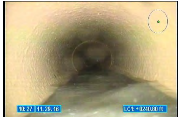
3940_ec63616d-3e23-4262-9e6d-2404daddbac9.jpg, 00:00:54, 241.40 Water Level, Sag in pipe
