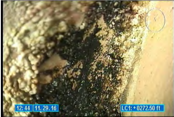
3660_2cf7b744-8154-4459-b376-09f52a36a021.jpg, 00:00:19, 272.50 Infiltration Stain, from 09 to 03 o'clock
