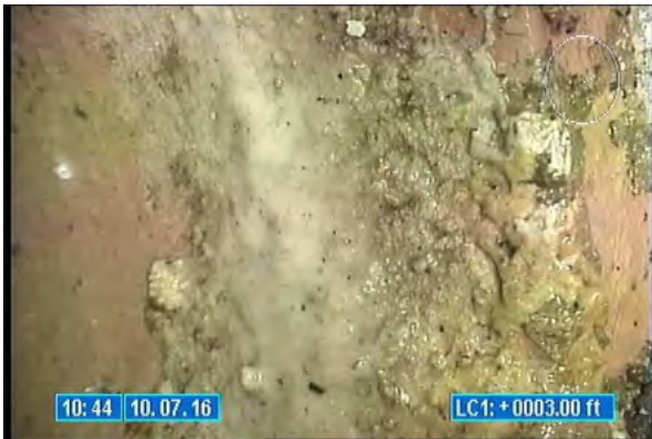
3500_2f890bac-0cc9-4340-adcb-2dd6acc17f3b.jpg, 00:00:01, 3.00 Deposits Attached Encrustation, from 07 to 05 o'clock, within 8 inch
