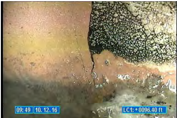
3560_5bcc1352-d9cf-4c88-96cb-6eb58bf5ae39.jpg, 00:00:54, 96.40 Fracture Multiple, from 12 to 12 o'clock, within 8 inch
