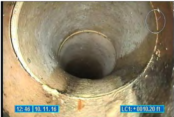
3620_2aee5511-02c4-4978-be2b-23ba9f513399.jpg, 00:00:05, 10.20 Tap Factory Made, at 02 o'clock, 6 inch dim
