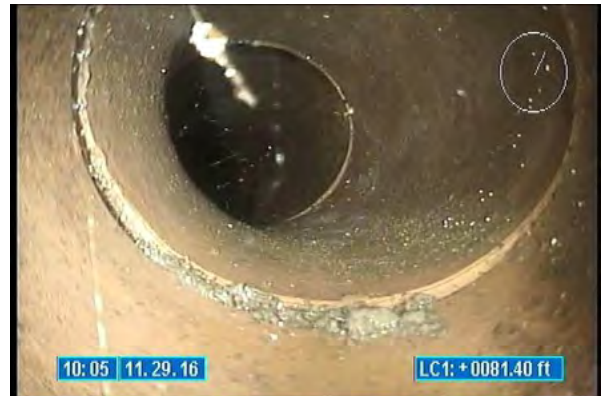
3940_bca7e39a-cfae-402c-a728-0e1459ba6836.jpg, 00:00:14, 81.40 Tap Factory Made, at 02 o'clock, 6 inch dim
