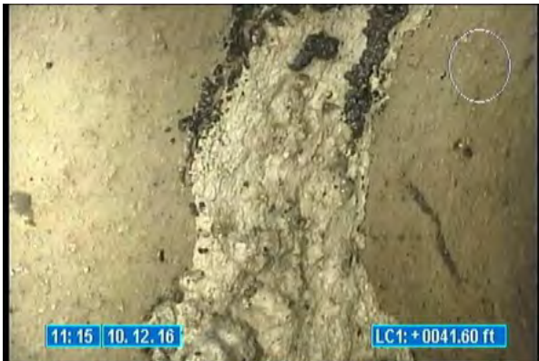
3690_2ba00e99-b2f0-432a-933e-555eee8c93e9.jpg, 00:00:11, 41.60 Deposits Attached Encrustation, from 08 to 04 o'clock, within 8 inch
