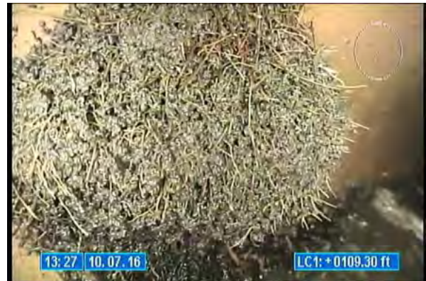
3410_322bd7f1-9474-4c2f-8bf6-c407b2eb2d01.jpg, 00:00:20, 109.30 Roots Medium Joint, at 07 o'clock, within 8 inch
