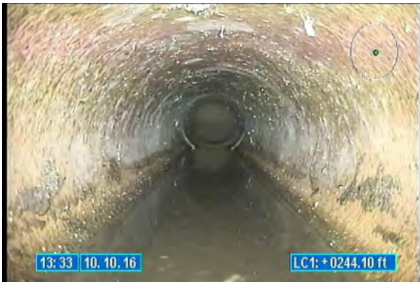
3310_93c8ffb4-fc37-4e16-8f04-93b6b5ea9371.jpg, 00:00:32, 244.10 Water Level, Sag in pipe
