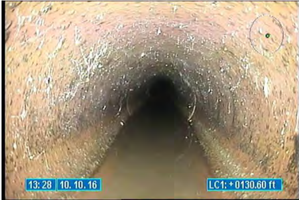
3310_aec7d82a-f7e2-410f-91be-ae04106e20ab.jpg, 00:00:22, 130.60 Water Level, Sag in pipe, S01
