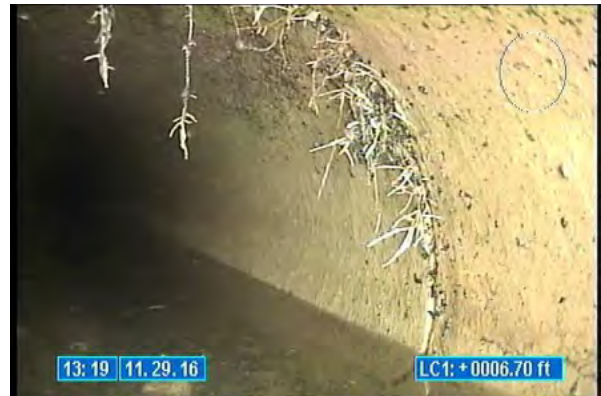
3870_daf9ae71-2bba-469b-8003-2733e61613a0.jpg, 00:00:02, 6.70 Roots Fine Joint, from 09 to 03 o'clock, within 8 inch
