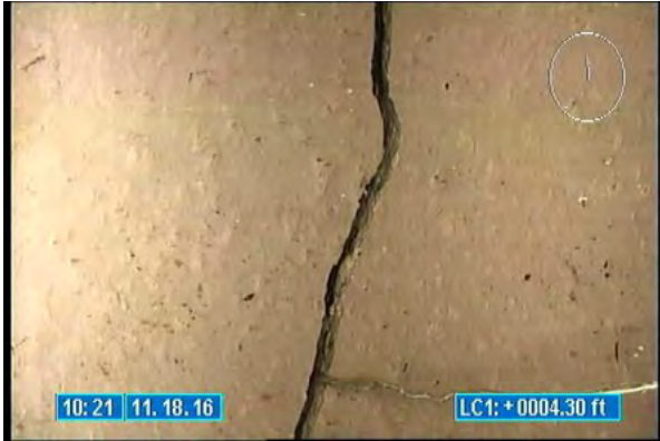
3350_d4b2a187-7a2f-4e7f-a82f-2a240d45ad36.jpg, 00:00:01, 4.30 Fracture Circumferential, from 12 to 12 o'clock, within 8 inch
