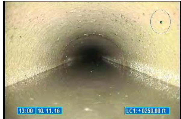
3620_b229f97c-598d-4536-9a7b-d69856782fcc.jpg, 00:00:40, 250.70 Water Level, Sag in pipe
