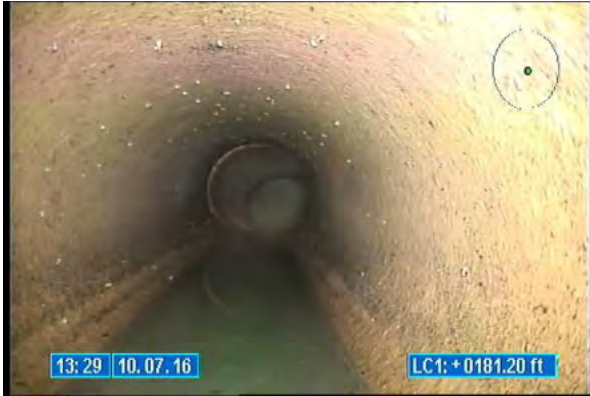
3410_eff85735-3d69-4b88-95d5-12269c2a54c2.jpg, 00:00:26, 181.10 Water Level, Sag in pipe
