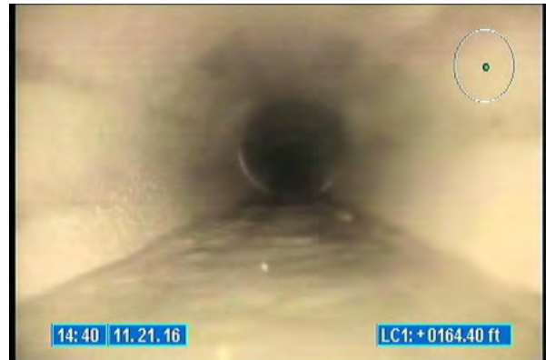
3750_9259c17a-3fb1-4d67-8fab-32df62b45b2c.jpg, 00:00:19, 164.50 Water Level, Sag in pipe
