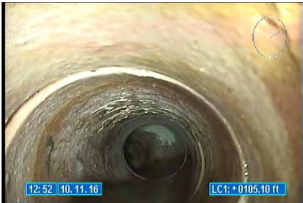
3620_cf8efdb9-eaad-48dc-a10d-1f7bb8d2f109.jpg, 00:00:20, 105.10 Infiltration Runner, at 02 o'clock, within 8 inch
