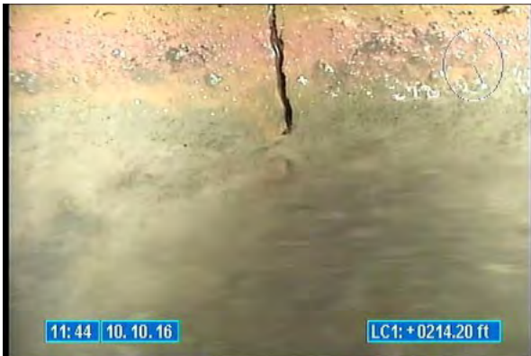
3300_8aa1ccb1-c1c9-4297-a74e-3dbf19d8dd77.jpg, 00:00:32, 214.20 Infiltration Gusher, at 06 o'clock
