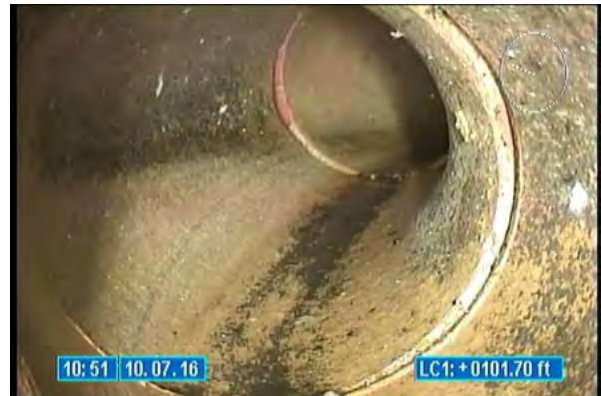
3500_a13ea253-2692-4ec3-9c42-3fdb08e682fd.jpg, 00:00:15, 101.70 Tap Factory Made Active, at 10 o'clock, 6 inch dim
