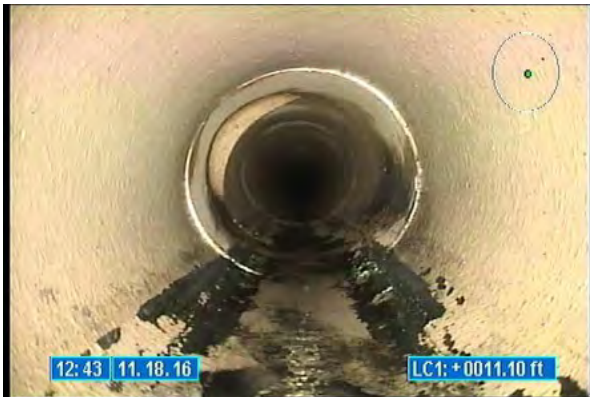
3210_96c3feb0-db38-4dd1-9241-f7ca90a7999d.jpg, 00:00:01, 11.10 Water Level, Sag in pipe
