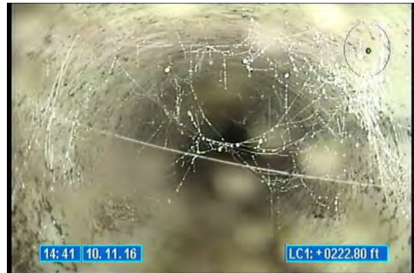
3540_a6fb6589-a6e1-420a-b164-ae40ab4efd6c.jpg, 00:00:36, 222.80 Water Level, Sag in pipe, F01
