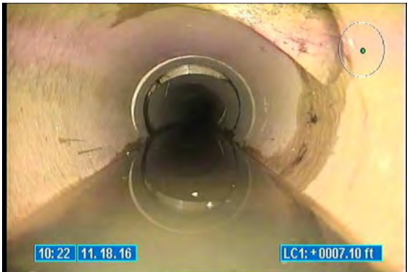
3350_26244ea5-4db7-4b50-aaff-0d593874cd54.jpg, 00:00:03, 7.10 Water Level, Sag in pipe
