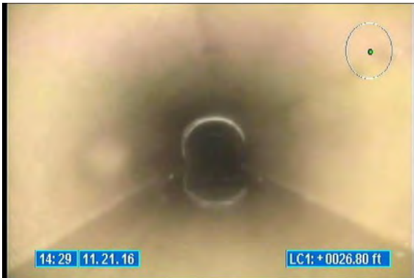
3750_5e0e665b-d286-4408-a6a2-e56a4ca11285.jpg, 00:00:05, 26.80 Water Level, Sag in pipe
