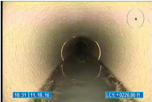
3350_d852944c-4d93-4429-9c03-d037154c891a.jpg, 00:00:23, 226.80 Water Level, Sag in pipe, S01
