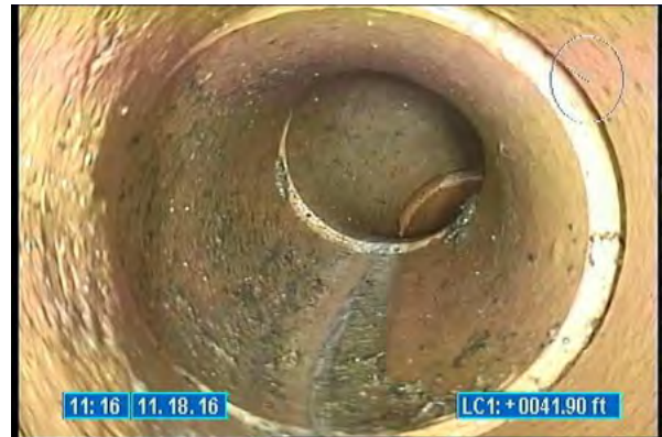
3430_070e7b54-14f2-4533-864c-ff3e975a4ca1.jpg, 00:00:03, 41.90 Tap Factory Made, at 10 o'clock, 6 inch dim
