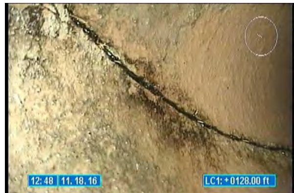
3210_361a2bdd-fd0c-409a-9991-b8c17da00235.jpg, 00:00:13, 128.00 Fracture Multiple, from 12 to 12 o'clock, within 8 inch
