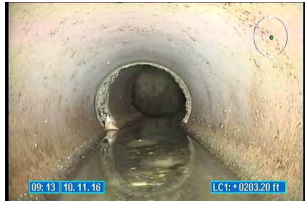
3100_9653e56d-d8da-48c3-9c63-70001441afb8.jpg, 00:00:24, 203.20 Water Level, Sag in pipe
