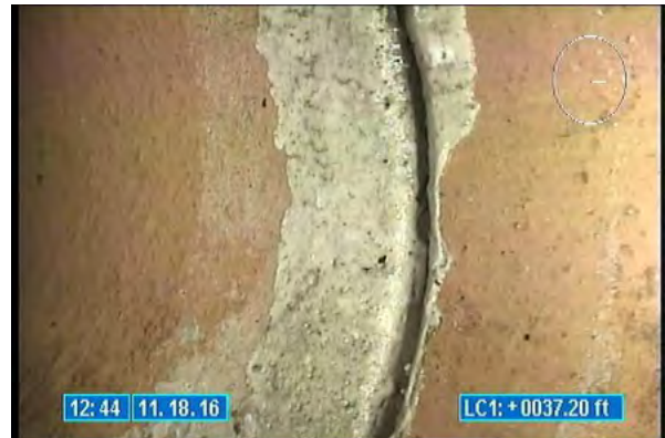
3210_d8a812dd-589b-4361-a852-3e2a480d76d7.jpg, 00:00:04, 37.20 Deposits Attached Encrustation, from 08 to 04 o'clock, within 8 inch
