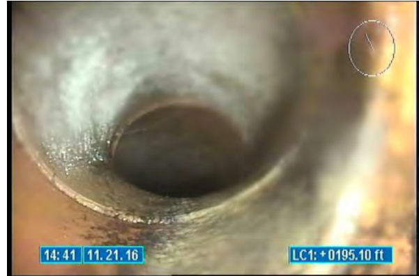
3750_bd50da92-0bdc-43a0-b8fd-aea83babced5.jpg, 00:00:22, 195.10 Tap Factory Made Active, at 11 o'clock, 6 inch dim
