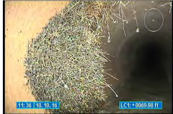
3300_c5178672-055c-4719-b3d7-966367c1b590.jpg, 00:00:13, 69.90 Roots Medium Joint, from 07 to 05 o'clock, within 8 inch
