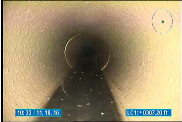
3350_94ab898b-328d-4709-be36-d07261f8b230.jpg, 00:00:28, 307.20 Water Level, Sag in pipe, S02
