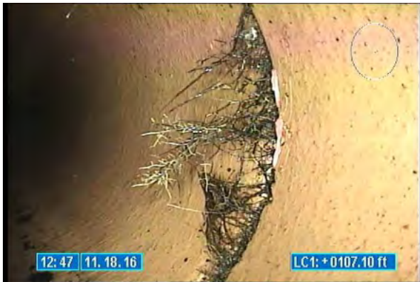
3210_8ada517f-5b95-41ab-ae9c-c71541db9d06.jpg, 00:00:10, 107.10 Roots Fine Joint, from 08 to 04 o'clock, within 8 inch
