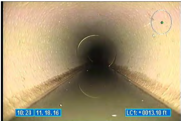
3350_331dcfa1-fc25-4757-8335-775d45f48723.jpg, 00:00:06, 13.10 Water Level, Sag in pipe
