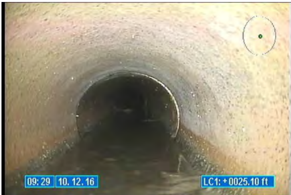
3560_37501c0a-8f5d-466c-bb7b-4eca425fc60e.jpg, 00:00:06, 25.10 Deposits Settled Gravel, at 06 o'clock, within 8 inch
