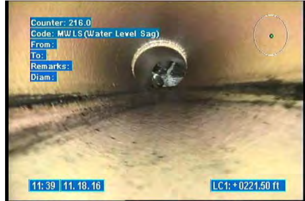
3430_7d187d8a-88e8-47c3-adcf-6d5b251520de.jpg, 00:00:35, 221.30 Water Level, Sag in pipe
