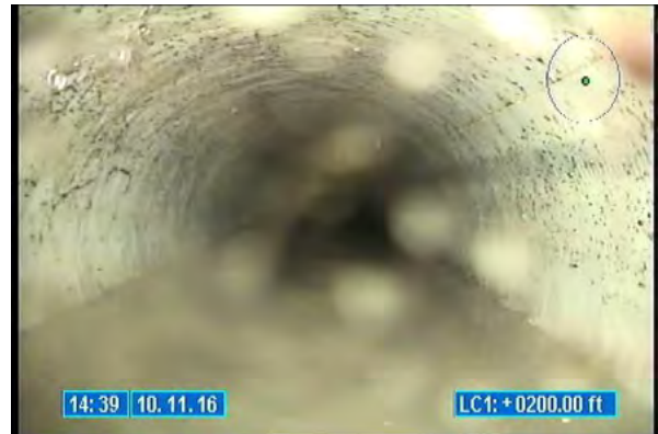
3540_92bae998-dfac-4f62-9919-eee192d4cd10.jpg, 00:00:33, 200.00 Water Level, Sag in pipe
