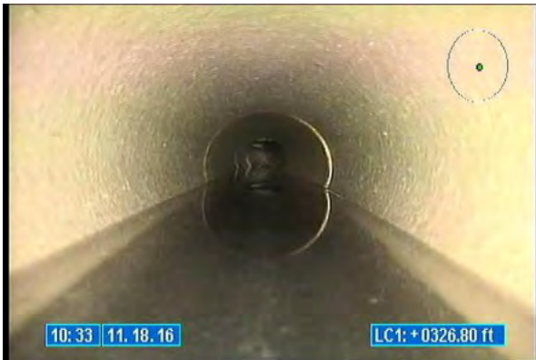
3350_4c0adbe2-6b45-40d9-bd9c-c069a7ebaa16.jpg, 00:00:30, 326.60 Water Level, Sag in pipe
