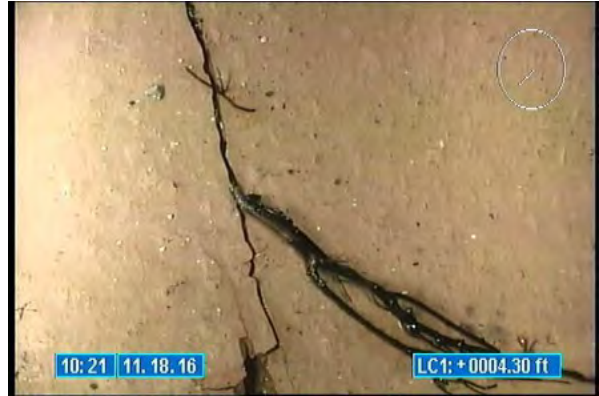
3350_0f779a2b-5d65-4469-80fb-41e30c44c82d.jpg, 00:00:02, 4.30 Roots Fine Joint, from 07 to 02 o'clock, within 8 inch
