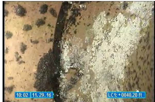
3940_d6cc5d3f-2c92-4faf-b469-af2ece6166f3.jpg, 00:00:07, 40.20 Deposits Attached Encrustation, from 08 to 04 o'clock, within 8 inch
