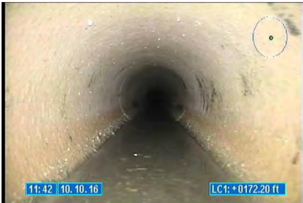
3300_5d526f15-2280-4f35-9c32-f4b782d449c4.jpg, 00:00:27, 172.20 Water Level, Sag in pipe
