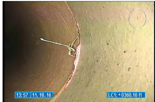
3180_a3db4632-351c-4a18-9708-bdc7e505ea3a.jpg, 00:00:33, 360.10 Roots Fine Joint, at 12 o'clock, within 8 inch
