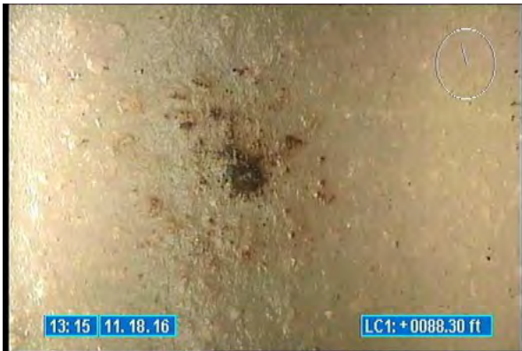
3190_fecdbc32-0e55-4093-8968-d4bcfd75c711.jpg, 00:00:09, 88.30 Infiltration Stain, at 11 o'clock
