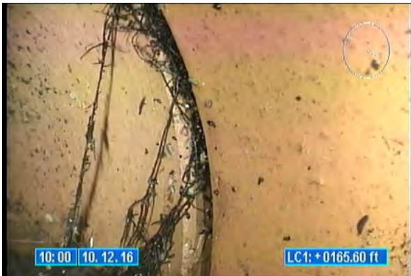
3560_c5a1e9ea-bd4e-4551-9524-9a2eed7bb003.jpg, 00:01:20, 165.60 Roots Fine Joint, from 08 to 04 o'clock, within 8 inch
