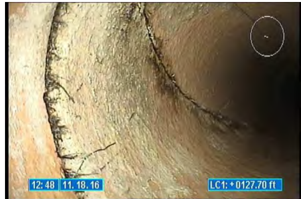
3210_a199ed30-16a3-4876-8a80-105724a74621.jpg, 00:00:12, 127.70 Deposits Attached Encrustation, from 07 to 05 o'clock, within 8 inch
