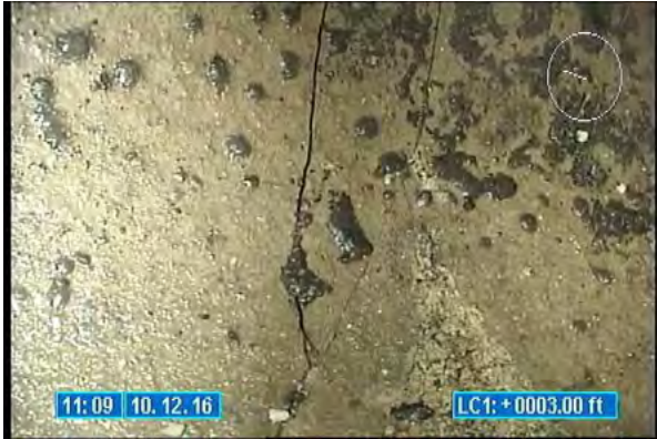
3690_ad5351fe-39c0-4759-a875-3176dfb53352.jpg, 00:00:01, 3.00 Fracture Circumferential, from 12 to 12 o'clock, within 8 inch
