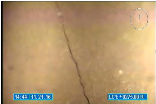
3750_0da8913e-5a90-42f3-8db3-ec0a9802aa68.jpg, 00:00:29, 275.00 Crack Circumferential, from 12 to 12 o'clock
