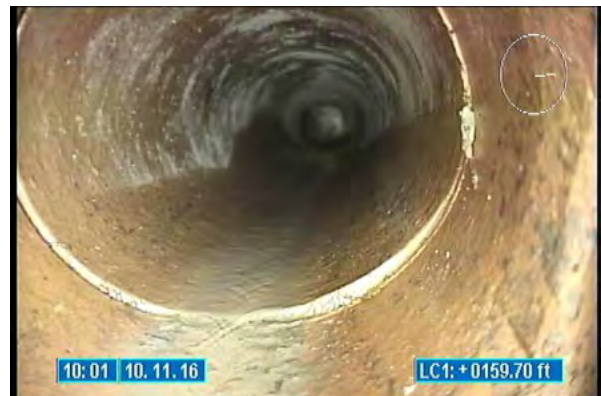
3120_a5146c70-94aa-4adb-b413-77b141f4fe4f.jpg, 00:00:27, 159.70 Tap Factory Made Active, at 03 o'clock, 6 inch dim
