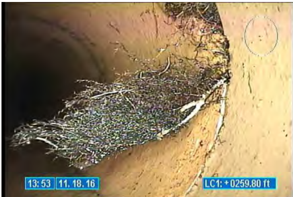
3180_0b98427e-3268-44f4-87be-d6a08218679e.jpg, 00:00:24, 259.80 Roots Medium Joint, from 07 to 05 o'clock, within 8 inch
