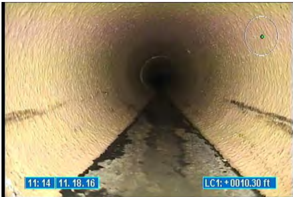
3430_db200f3a-c9b3-4eef-bbaf-37aabdfe6d23.jpg, 00:00:01, 10.30 Water Level, Sag in pipe
