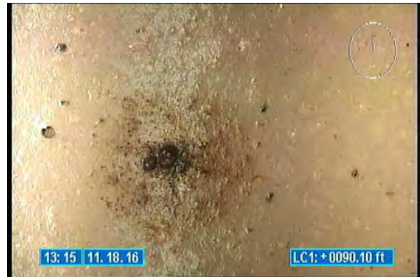
3190_65bf15b3-782f-44a2-8b05-f6b42adbbc24.jpg, 00:00:09, 90.10 Infiltration Stain, at 12 o'clock
