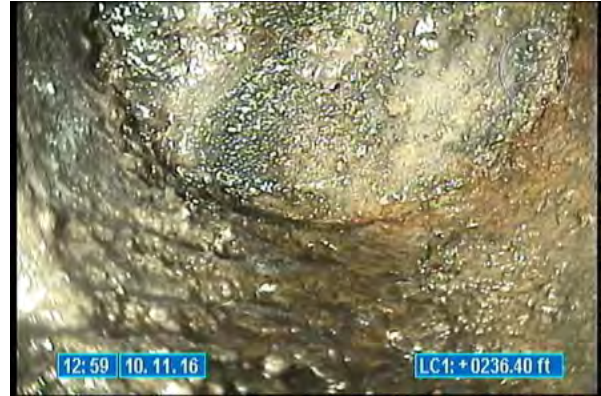
3620_8cdaed4e-3dba-40ee-9184-ecd8cbf470d2.jpg, 00:00:38, 236.40 Infiltration Stain, at 10 o'clock
