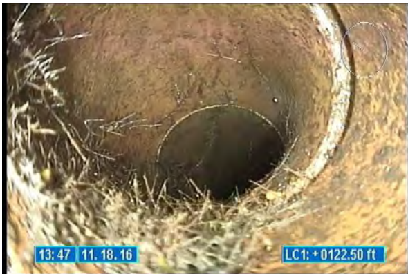
3180_566cc142-7146-4ccb-8d86-11cde8e7edf7.jpg, 00:00:11, 122.50 Tap Factory Made, at 10 o'clock, 6 inch dim
