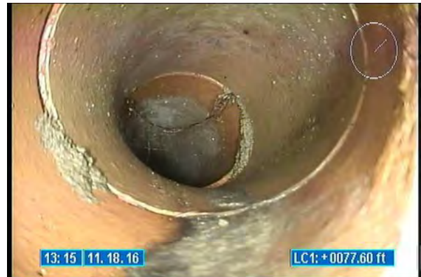
3190_aa7518c0-eac8-4cf4-94c9-26810b331fe1.jpg, 00:00:07, 77.60 Tap Factory Made, at 02 o'clock, 6 inch dim
