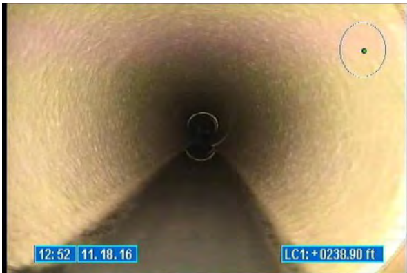
3210_c67f142a-f207-459c-ba56-ddbe3545cbc7.jpg, 00:00:21, 239.00 Water Level, Sag in pipe
