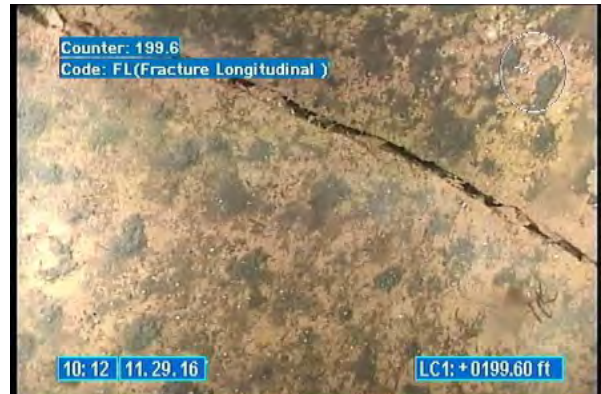
3940_8c856fc8-0c6d-4460-aef8-0f6d2132eed.jpg, 00:00:32, 199.60 Fracture Longitudinal, at 10 o'clock, within 8 inch
