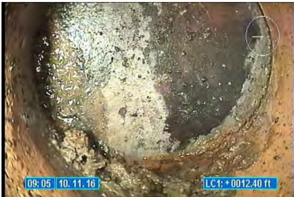
3100_01d15003-ecdc-4a04-a77e-02e4276afe36.jpg, 00:00:05, 12.40 Tap Factory Made Capped, at 09 o'clock, 6 inch dim
