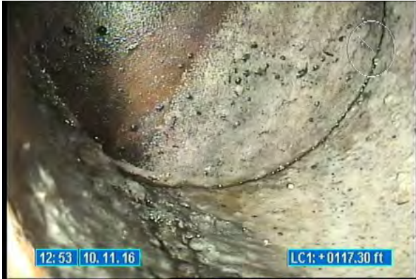
3620_1f6d6054-043b-4d45-a81f-d23ad4939f3c.jpg, 00:00:23, 117.30 Infiltration Stain, at 10 o'clock
