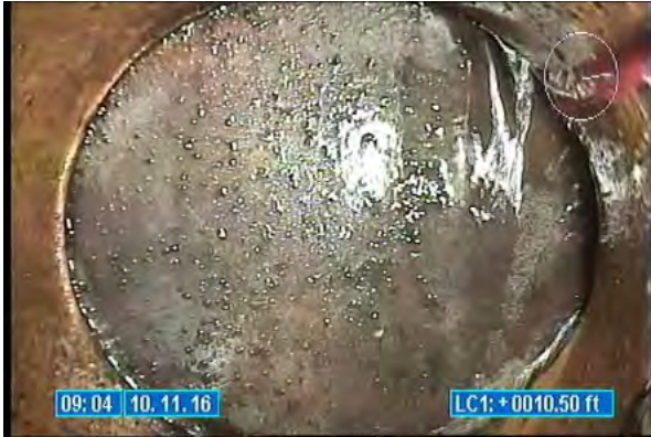
3100_0d1c0256-cf5a-4922-b386-0cb665322655.jpg, 00:00:02, 10.50 Tap Factory Made Defective, at 03 o'clock, 6 inch dim
