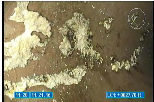
3280_c07432bd-4926-4b00-b1e1-0cbdc7851953.jpg, 00:00:03, 27.70 Deposits Attached Encrustation, from 11 to 01 o'clock
