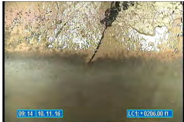
3100_5f6b24e2-a924-4add-966b-d66c8fe27095.jpg, 00:00:27, 206.00 Fracture Circumferential, from 04 to 06 o'clock, within 8 inch
