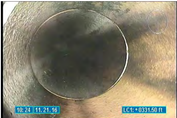
3450_dbb99722-3d6d-4e39-acee-c1b7605ff936.jpg, 00:00:43, 331.50 Tap Factory Made, at 06 o'clock, 6 inch dim
