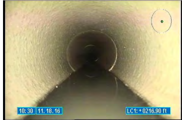
3350_6f523ad1-c221-4b5f-89ea-cdb16420d5ff.jpg, 00:00:22, 217.10 Water Level, Sag in pipe
