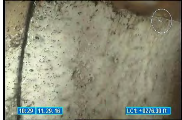
3940_cae37ef3-dce0-466b-bdd0-e28e3a322bea.jpg, 00:00:57, 276.30 Deposits Attached Encrustation, from 07 to 11 o'clock, within 8 inch
