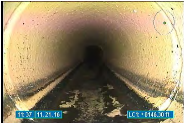
3290_f032c9f8-93c8-4872-9156-d49f686d544e.jpg, 00:00:19, 146.30 Water Level, Sag in pipe, S01
