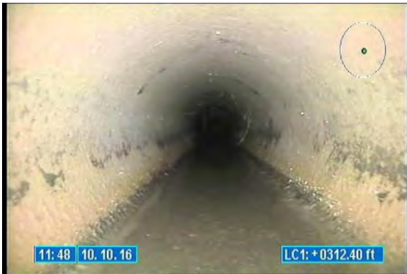
3300_438749d7-13bf-4b96-94a6-cf39c178c0a3.jpg, 00:00:41, 312.50 Water Level, Sag in pipe
