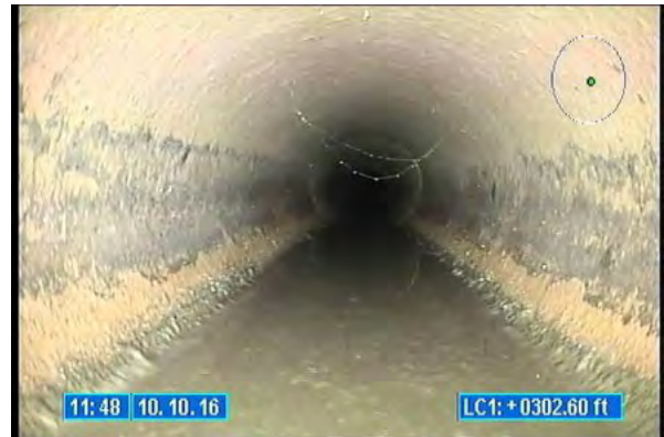
3300_a0e1744b-f921-4aba-a9d7-a6c41f30396b.jpg, 00:00:40, 302.60 Water Level, Sag in pipe
