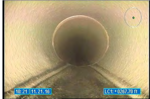
3450_f1dea24a-a1f5-4b3a-bc54-691e574861ca.jpg, 00:00:35, 267.80 Water Level, Sag in pipe
