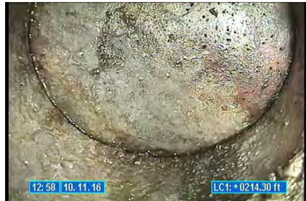
3620_0510000d-769a-4db4-86c5-32b760e7c4e8.jpg, 00:00:34, 214.30 Tap Factory Made Capped, at 02 o'clock, 6 inch dim
