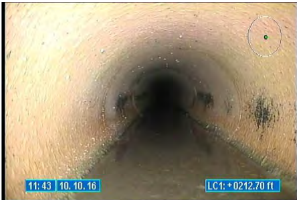
3300_e51eb558-4776-4ca2-86e3-f5f814a43b67.jpg, 00:00:30, 212.70 Deposits Settled Gravel, at 06 o'clock
