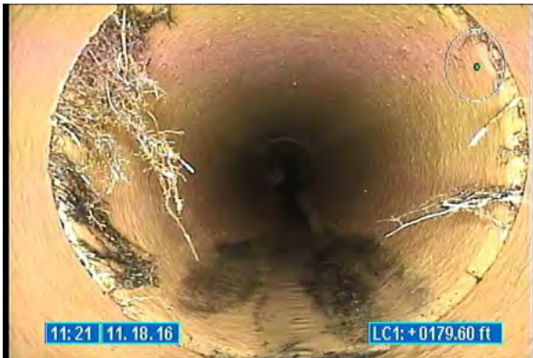
3430_dc3c9709-296b-4eca-876b-b88f237f14ca.jpg, 00:00:16, 179.60 Roots Medium Joint, from 07 to 05 o'clock, within 8 inch
