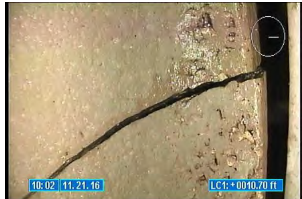
3450_59b8cba1-520e-4298-b6e8-a2dfe49f743d.jpg, 00:00:03, 10.70 Fracture Multiple, from 03 to 07 o'clock, within 8 inch
