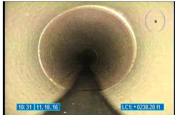
3350_7a3f1223-7c9f-43b6-ac04-466e91dc73bb.jpg, 00:00:24, 238.40 Water Level, Sag in pipe, F01
