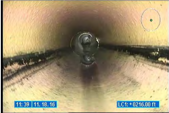
3430_c9d63cd6-bbc7-481d-8e40-95e9a479d759.jpg, 00:00:35, 216.00 Water Level, Sag in pipe
