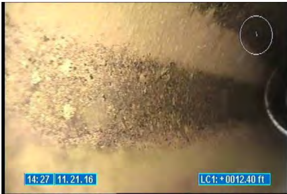
3750_cd4a52d2-4c81-4c3f-9d13-e15f094b1340.jpg, 00:00:02, 12.50 Water Level, Sag in pipe
