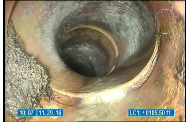
3940_6ce4164c-6714-4dc9-bbf0-952e4e253a20.jpg, 00:00:19, 105.50 Tap Factory Made Active, at 02 o'clock, 6 inch dim
