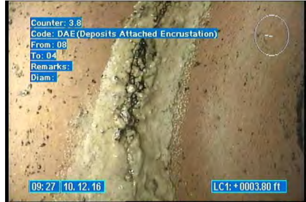
3560_75fa6616-943f-4ef8-90de-d25695fa0218.jpg, 00:00:02, 3.80 Infiltration Stain, from 08 to 04 o'clock, within 8 inch
