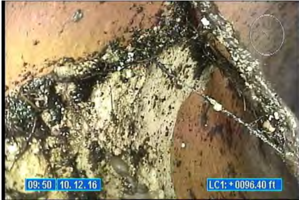
3560_e736aaa8-007f-4d2e-83de-0b7606db2ee1.jpg, 00:00:55, 96.40 Infiltration Stain, from 08 to 04 o'clock
