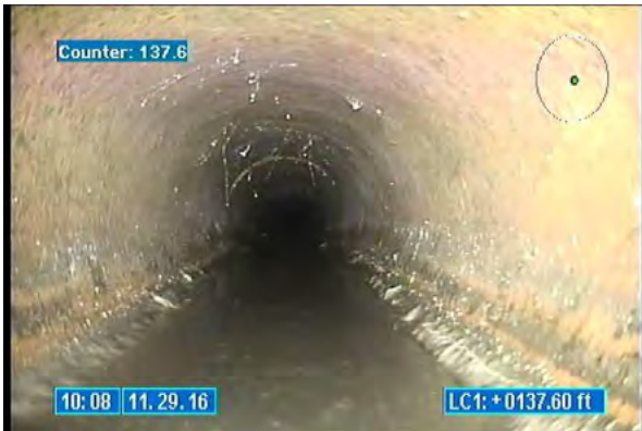
3940_fbd9f18c-71b1-4fe2-a828-b0a7689b847d.jpg, 00:00:22, 137.60 Water Level, Sag in pipe
