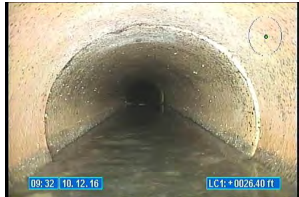
3560_34b0a8cb-8e10-42c8-8739-9eea4adff4d6.jpg, 00:00:11, 26.40 Deposits Settled Gravel, at 06 o'clock, within 8 inch
