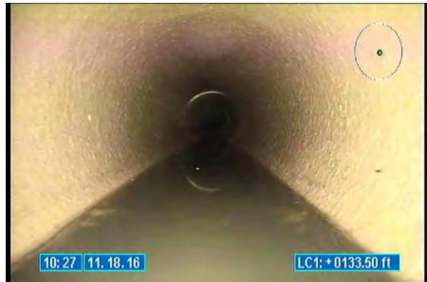
3350_4735eb51-50d1-4a7a-bcee-f5369ec0c387.jpg, 00:00:15, 134.00 Water Level, Sag in pipe
