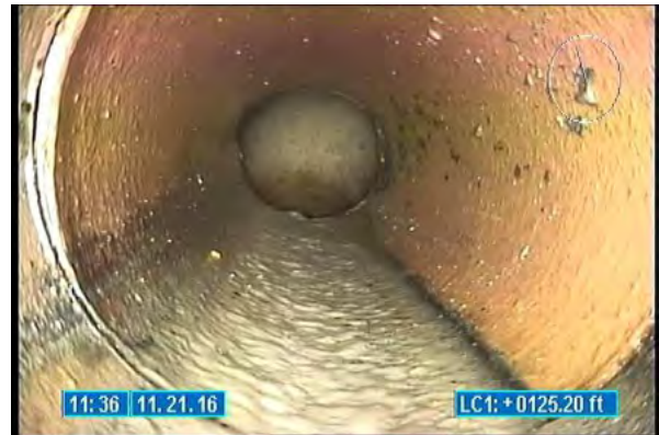
3290_7ac31017-401f-4164-9682-b07387f599b5.jpg, 00:00:17, 125.20 Tap Factory Made Active, at 11 o'clock, 6 inch dim
