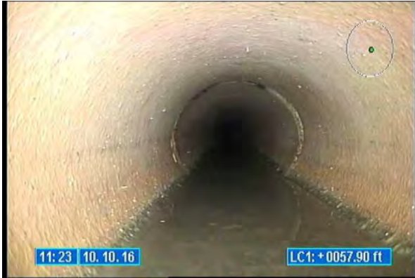
3300_4c1be84f-20cc-4472-8f3e-679a527da3b6.jpg, 00:00:07, 57.90 Deposits Settled Gravel, at 06 o'clock
