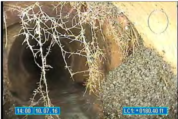
3230_4f540b86-00dd-4b29-8447-c42528393716.jpg, 00:00:20, 180.40 Roots Medium Joint, from 07 to 05 o'clock, within 8 inch
