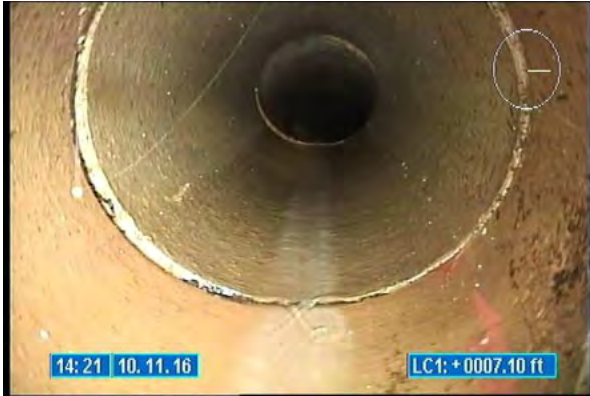
3540_086046a7-eb4e-47e2-aabe-928e0cc6f971.jpg, 00:00:01, 7.10 Tap Factory Made, at 03 o'clock, 6 inch dim
