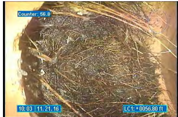
3450_0e94781a-f801-4ddd-ace5-63a945e8afae.jpg, 00:00:07, 56.80 Tap Factory Made Defective, at 10 o'clock, 6 inch dim
