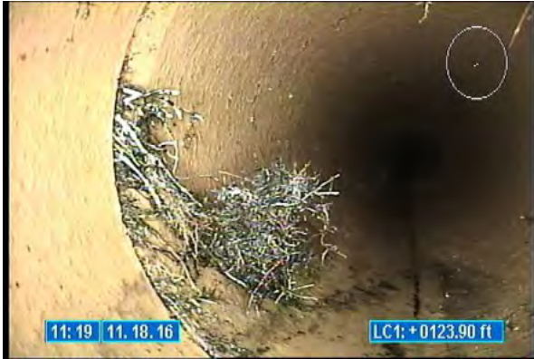
3430_ff2d6d6e-9907-4fa9-9ecb-18f0861c171e.jpg, 00:00:12, 123.90 Roots Medium Joint, from 07 to 05 o'clock, within 8 inch
