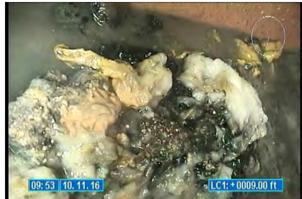
3120_48a35921-f667-4afa-bf75-a0f8ddce0925.jpg, 00:00:08, 9.00 Deposits Settled Other, at 06 o'clock
