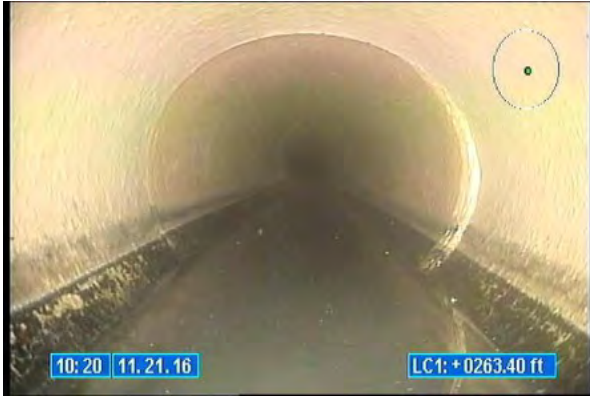
3450_ebf1b9b9-62d5-4974-bb09-63b72260be68.jpg, 00:00:35, 263.40 Water Level, Sag in pipe
