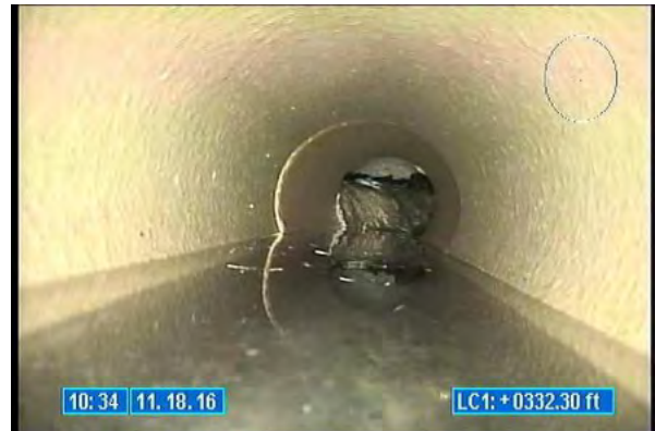
3350_acb3f889-3578-4a24-ba31-9a7fcdc7a50e.jpg, 00:00:30, 332.40 Water Level, Sag in pipe
