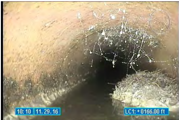
3940_109c41e6-c040-4842-bd77-d3852f18f1ff.jpg, 00:00:26, 166.00 Deposits Settled Gravel, at 06 o'clock
