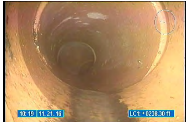
3450_4f775aba-ca21-4437-b2ce-70962c255d72.jpg, 00:00:32, 238.30 Tap Factory Made, at 10 o'clock, 6 inch dim
