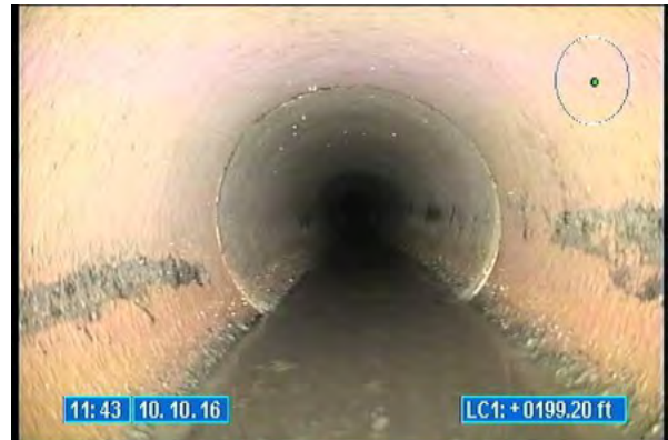
3300_bdc799ee-640c-46d7-a42f-8cd18fa94470.jpg, 00:00:29, 199.30 Water Level, Sag in pipe
