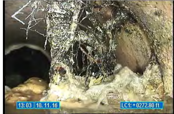
3620_6f8ed916-e783-445b-b644-d1e16970e776.jpg, 00:00:46, 272.80 Roots Medium Joint, from 01 to 05 o'clock, within 8 inch
