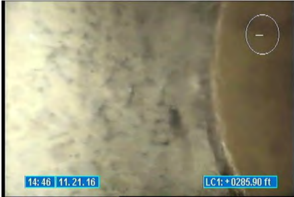
3750_bc13b1a0-decf-41f5-bfb1-e53fb28dfdb4.jpg,00:00:32, 285.90 Deposits Attached Encrustation, from 07 to 05 o'clock, within 8 inch
