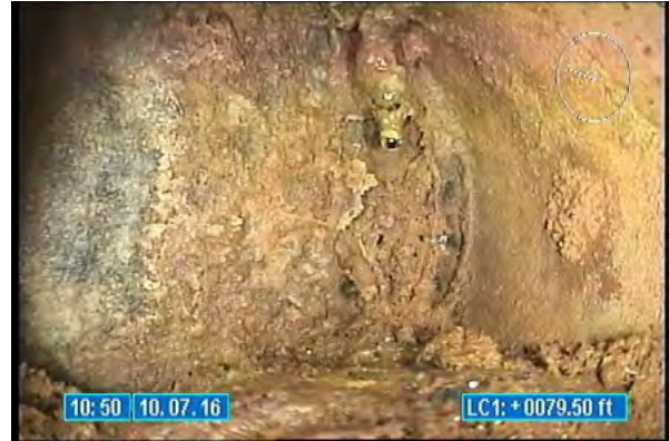
3500_9786b028-762c-4273-a3c4-64a9e31a3a60.jpg, 00:00:12, 79.50 Infiltration Dripper, at 10 o'clock
