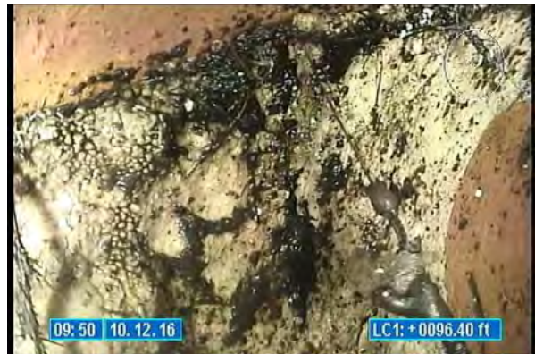
3560_2c32a0c7-36ac-4c0a-a829-b47f893b4d73.jpg, 00:00:55, 96.40 Deposits Attached Encrustation, from 07 to 05 o'clock
