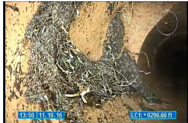
3180_bb3c383d-2509-4cb7-b544-70f37835ec70.jpg, 00:00:19, 206.60 Roots Medium Joint, from 07 to 05 o'clock, within 8 inch
