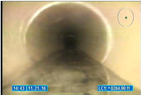
3750_b17e39fd-c3f1-4c2e-829e-688db773d6b6.jpg, 00:00:28, 264.90 Water Level, Sag in pipe
