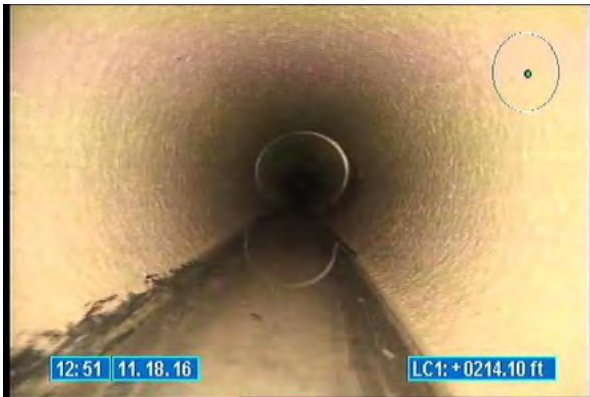
3210_63610f0f-139e-4dcc-b57d-7a7d3050779b.jpg, 00:00:18, 214.50 Water Level, Sag in pipe
