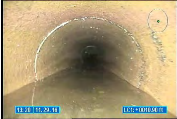
3870_93be6e96-702a-4811-8586-a4457c1869b4.jpg, 00:00:02, 10.90 Water Level, Sag in pipe
