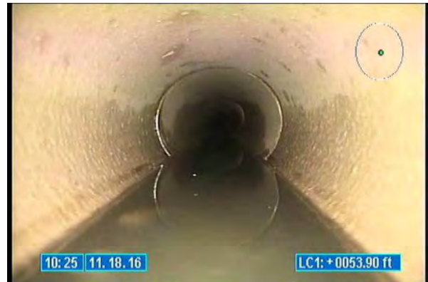
3350_e1091a3d-1d12-4845-9132-b4ae0f79dbbc.jpg, 00:00:08, 53.80 Water Level, Sag in pipe
