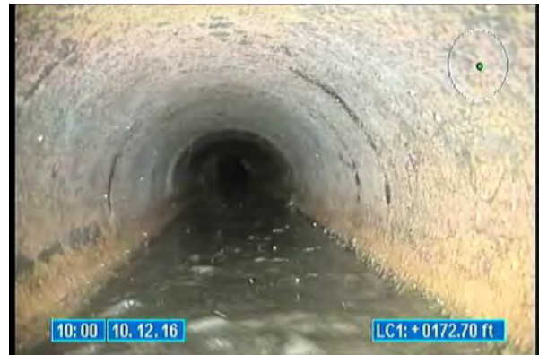
3560_d870a9eb-27d8-4fe8-b1fe-ac59f8194a38.jpg, 00:01:21, 172.70 Deposits Settled Gravel, at 06 o'clock
