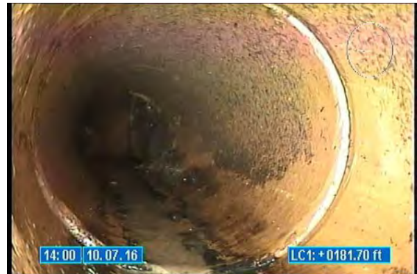
3230_5f2a1e4b-63fa-42eb-b7b4-f98d95ddc609.jpg, 00:00:20, 181.70 Tap Factory Made Active, at 09 o'clock, 6 inch dim
