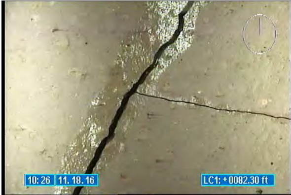
3350_36196537-7552-4243-9398-677411a86415.jpg, 00:00:11, 82.30 Fracture Multiple, from 12 to 12 o'clock, within 8 inch
