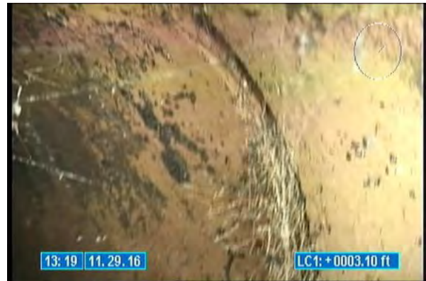
3870_e4f826b3-7fbe-4c5c-80bd-408ce021ebc6_20170412_133558_814.jpg, 00:00:00, 0.00 Water Level
