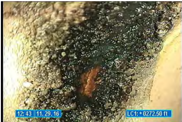
3660_d8507451-8d32-4c78-b2a0-4bfdca2bdea9.jpg, 00:00:19, 272.50 Crack Circumferential, from 09 to 03 o'clock
