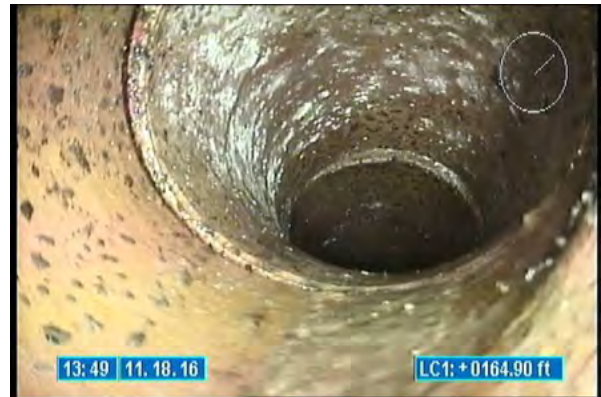
3180_d5fc1eb0-c45e-4c89-997a-f27dae5d158e.jpg, 00:00:14, 164.90 Tap Factory Made, at 02 o'clock, 6 inch dim
