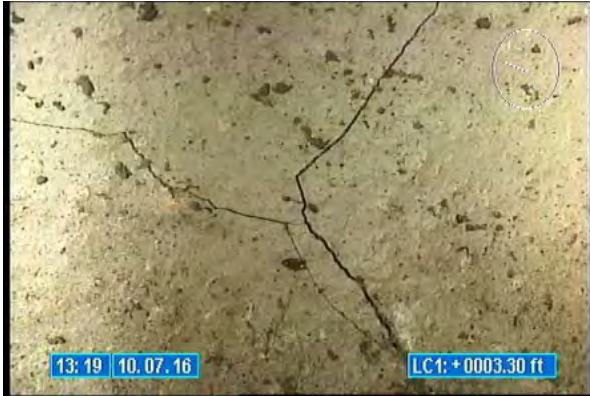
3410_33ad65c3-c5aa-4836-9b66-d9abecae31d8.jpg, 00:00:01, 3.30 Crack Multiple, from 07 to 05 o'clock
