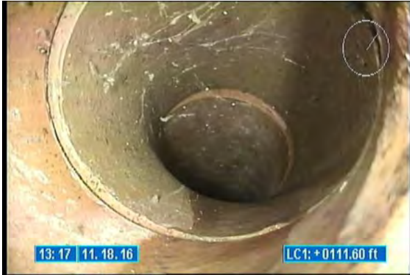
3190_a7b7a810-739b-4b98-99db-ae8d6a5dbb49.jpg, 00:00:13, 111.60 Tap Factory Made, at 02 o'clock, 6 inch dim
