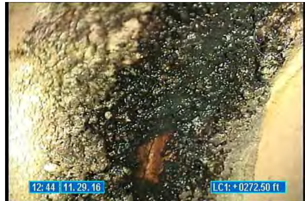
3660_463f702c-f6af-4eeb-8181-abc10c0ae744.jpg, 00:00:19, 272.50 Deposits Attached Encrustation, from 09 to 03 o'clock
