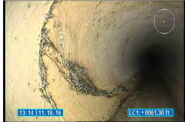
3190_e4129c58-a1e6-4c82-9329-428f87cf4de6.jpg, 00:00:05, 61.30 Roots Fine Joint, at 09 o'clock, within 8 inch
