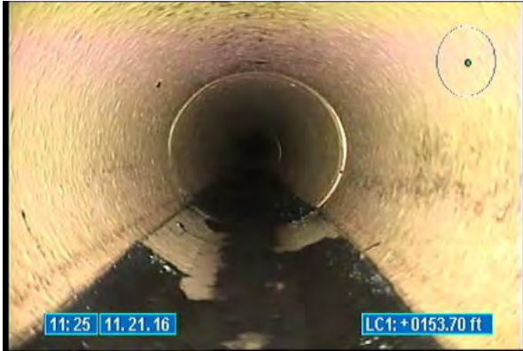
3280_32a35a7b-e931-48f7-8ca2-1d3ce0112bc7.jpg, 00:00:15, 153.70 Water Level, Sag in pipe, S01
