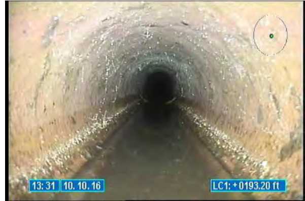
3310_56c59044-c4f3-437d-86c2-7cc57f153a70.jpg, 00:00:28, 193.40 Water Level, Sag in pipe
