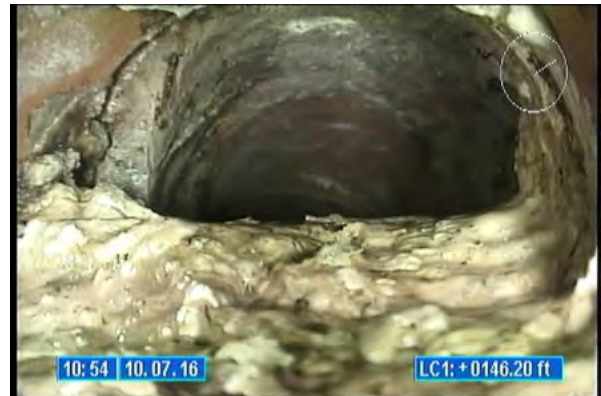
3500_29c6ff5d-0b9c-43b6-8cc8-abd14ab4a076.jpg, 00:00:22, 146.20 Tap Factory Made Defective, at 03 o'clock, 6 inch dim
