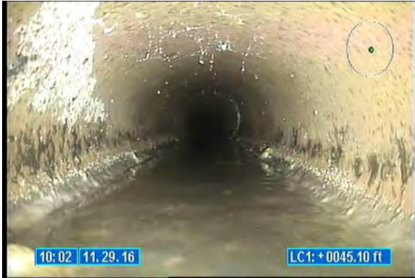
3940_e8bd78d2-7ade-4fa1-9acf-e6dccc31b785.jpg, 00:00:08, 45.10 Water Level, Sag in pipe
