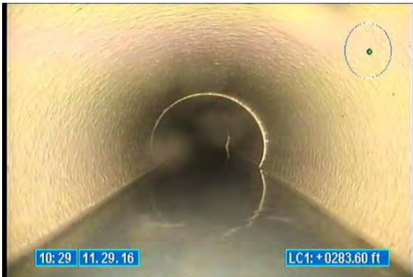
3940_ba2382ff-7990-41d2-adc7-b1f66891b3c1.jpg, 00:00:58, 283.60 Water Level, Sag in pipe
