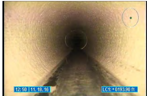
3210_51ffd84a-5f82-4e95-8892-11275f7aca04.jpg, 00:00:17, 193.90 Water Level, Sag in pipe
