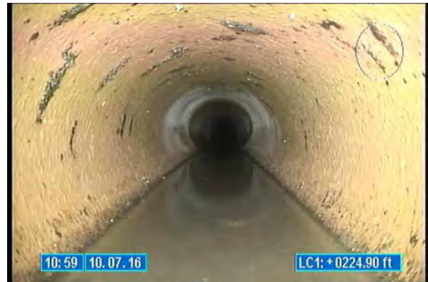
3500_f4a4d7c5-0ab3-47e9-b6a7-4fd1a2f2b9b0.jpg, 00:00:33, 224.90 Water Level, Sag in pipe
