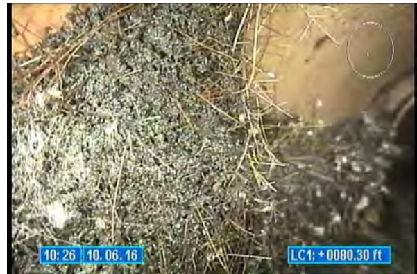
3010_96e0badc-32bc-4bb3-b9bc-9b9ac733ed29.jpg, 00:00:09, 80.30 Roots Medium Joint, at 08 o'clock, within 8 inch
