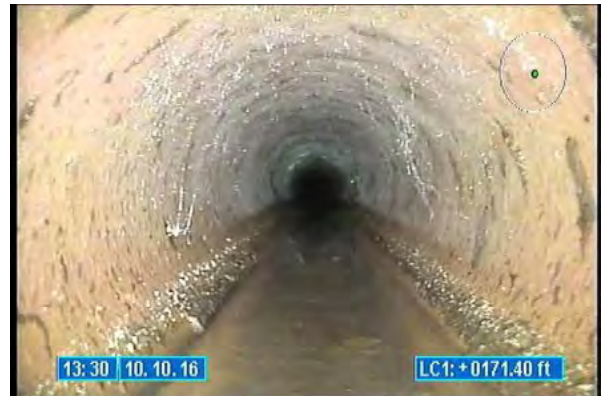
3310_a3b703a4-2e3c-42f1-beed-08048399a0c2.jpg, 00:00:26, 171.60 Water Level, Sag in pipe
