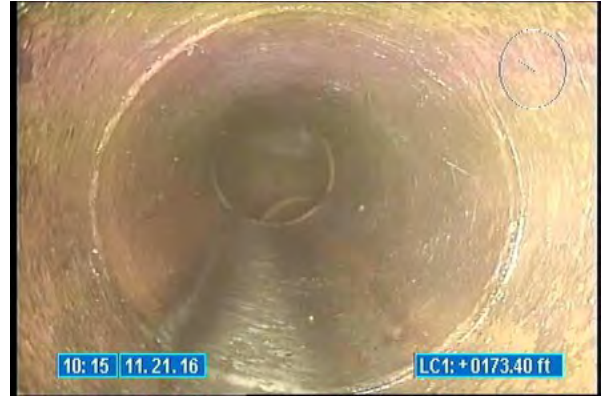
3450_6ca00d96-a211-40a1-b068-de65cdf635.jpg, 00:00:23, 173.40 Tap Factory Made, at 10 o'clock, 6 inch dim
