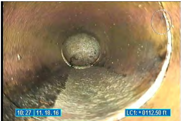
3350_d7af9a17-3b25-49cc-8f0a-2a3e0fc9a5f0.jpg, 00:00:14, 112.50 Tap Factory Made, at 11 o'clock, 6 inch dim
