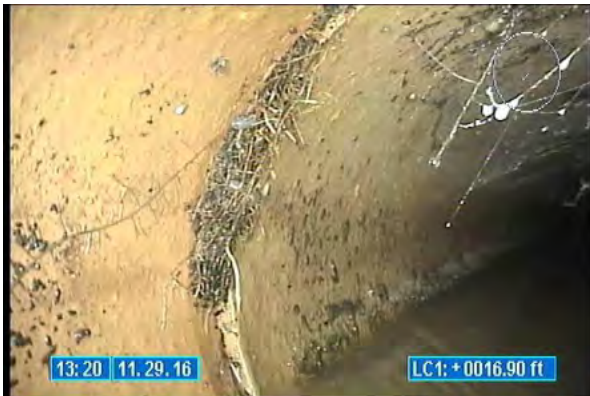
3870_b2f920b0-de13-4794-b6af-a4c76d0b66f8.jpg, 00:00:04, 16.90 Roots Fine Joint, from 08 to 03 o'clock, within 8 inch
