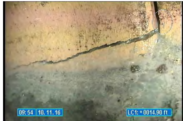
3120_1903ecb3-9165-4d92-ac8b-10d537d11756.jpg, 00:00:12, 14.90 Fracture Longitudinal, at 05 o'clock, within 8 inch
