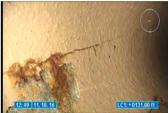
3210_ec9192d1-964c-4215-81c8-a59c2b88123d.jpg, 00:00:14, 131.00 Infiltration Stain, from 06 to 10 o'clock
