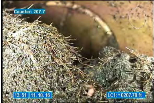
3180_ae6207fe-7e5d-4deb-864f-1c447184553b.jpg, 00:00:20, 207.70 Tap Factory Made, at 10 o'clock, 6 inch dim
